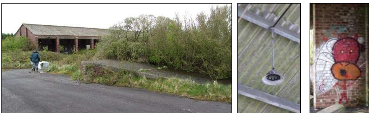
Figure 62. Standing remains of the domestic site for Hartland Radar station, MDV72114, including fixtures and fittings and recent graffiti. Photographs: Stephanie Knight
