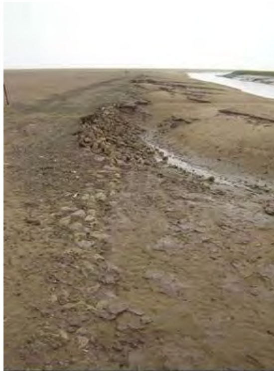
Plate 2 Eroding causeway (SH22), Saltfleet Haven, Skidbrooke with Saltfleet
