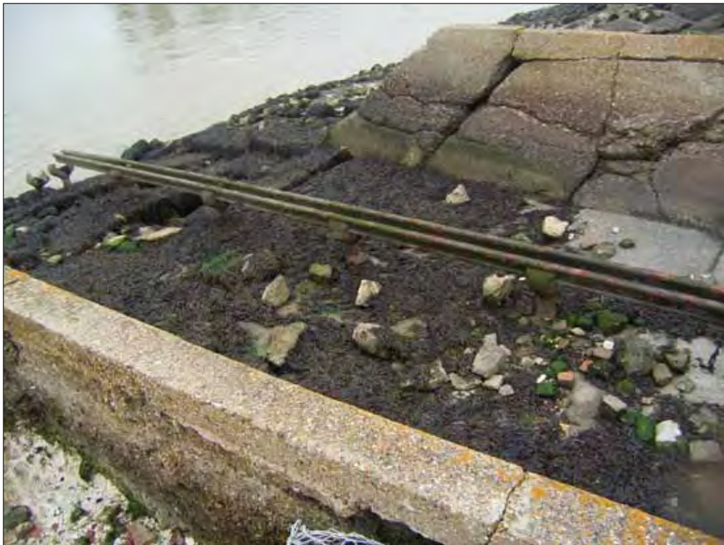
Plate 8: Higham Stretch, the Brennan torpedo installation at Cliffe Fort (TQ 77 NW 1015). Many of the fittings are still in situ.
