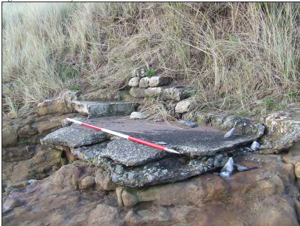
Fig 5.12.9 eroding concrete structure built utilising concrete sandbags, possibly of Second World War date.
