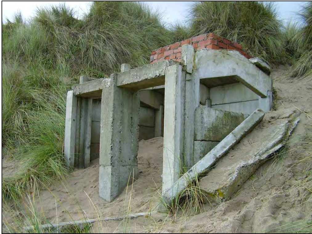
Fig 5.8.16 eroding military structure.
