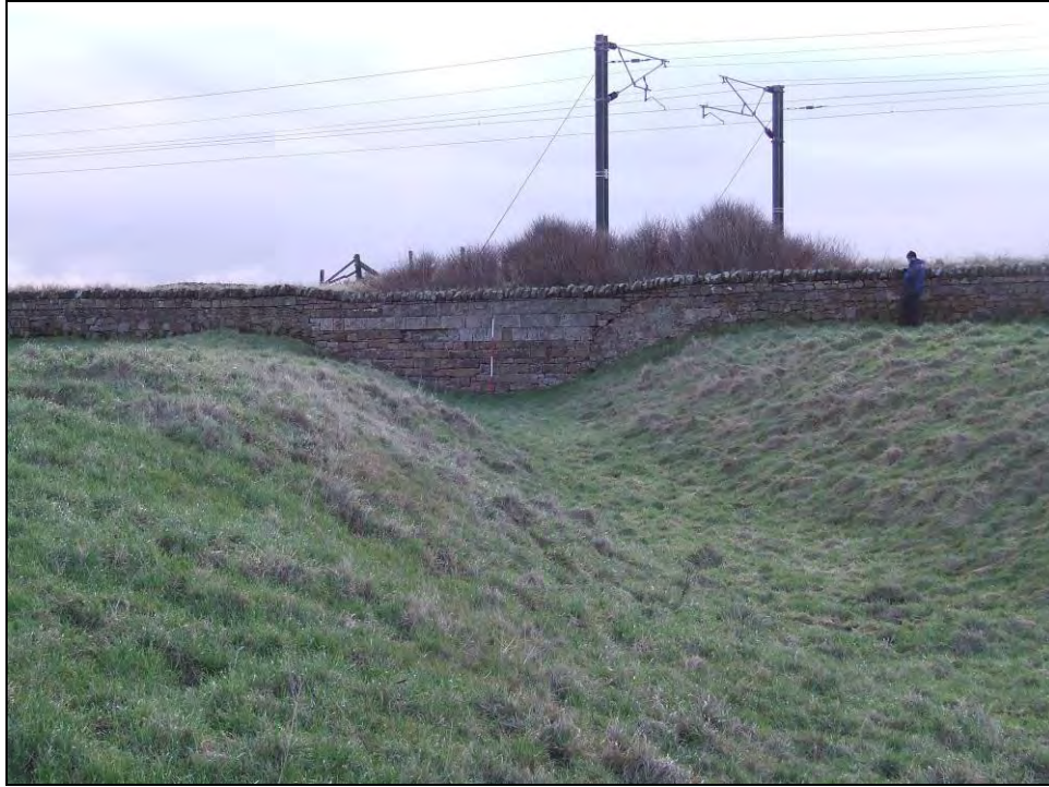
Fig 5.12.5 The former railway cutting, showing the modern route of the line behind the stone wall.
