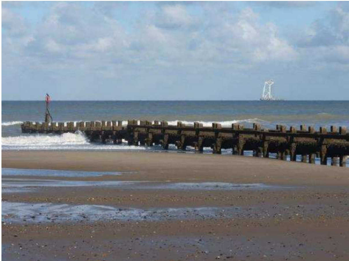
Figure 9. Gas pipeline along groyne at Bacton, with Windfarm development in the background
