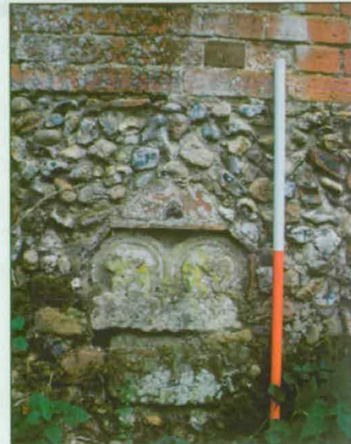
Plate 28: Re-used stone from the abbey (02a) set into the north-facing wall of an agricultural building adjacent to Tilty Mill
