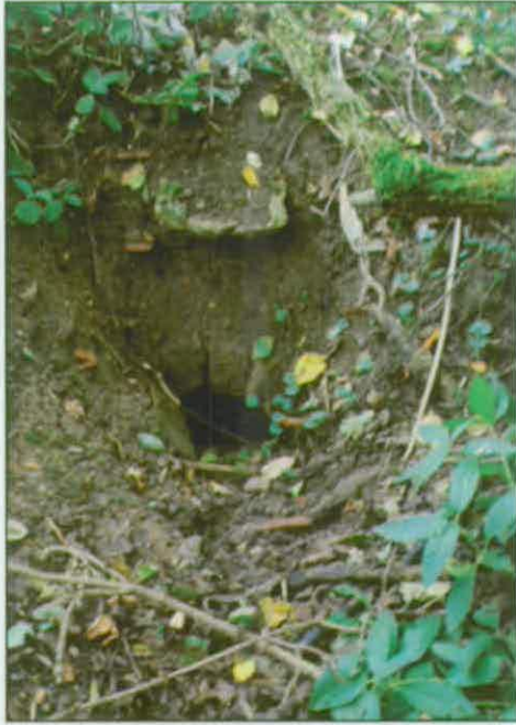
Plate 11: Culvert (28) beneath flint and brick building adjacent to Tilty Mill, from west
