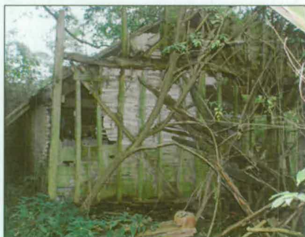
Plate 10: Collapsed timber framed building (28a) close to Tilty Mill, from south-west
