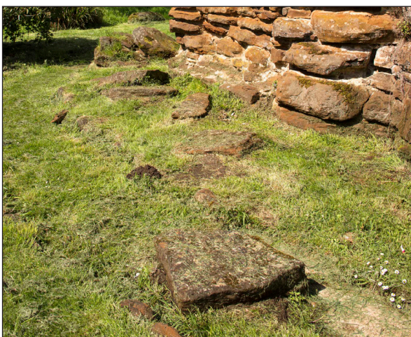
Fig. 21 (above) Loose stones outside the Bath House (© Historic England, Patricia Payne DP232119)
