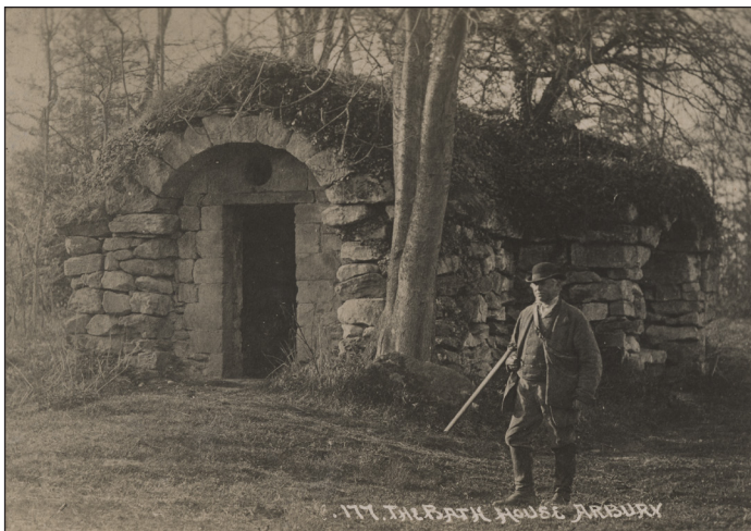
Fig. 42 The bath house at Arbury Hall, Warwickshire, mid- to late 18 th -century in date (Warwickshire County Record Office PH 352/63/41)
