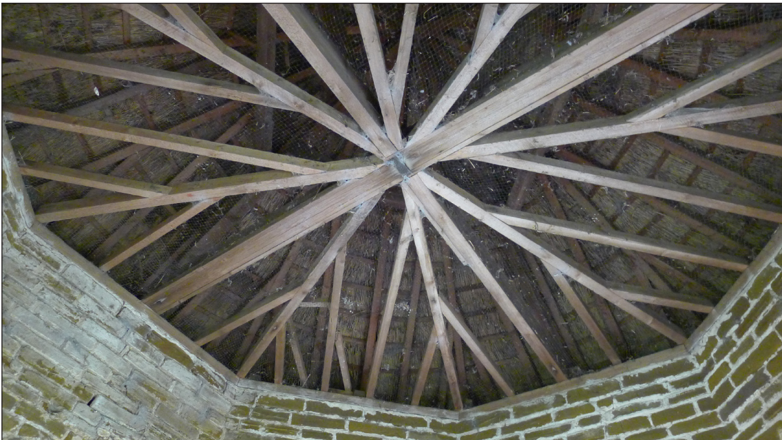
Fig. 11 The roof structure of the northern room of the Bath House, seen from below (© Historic England, Jonathan Kewley)
