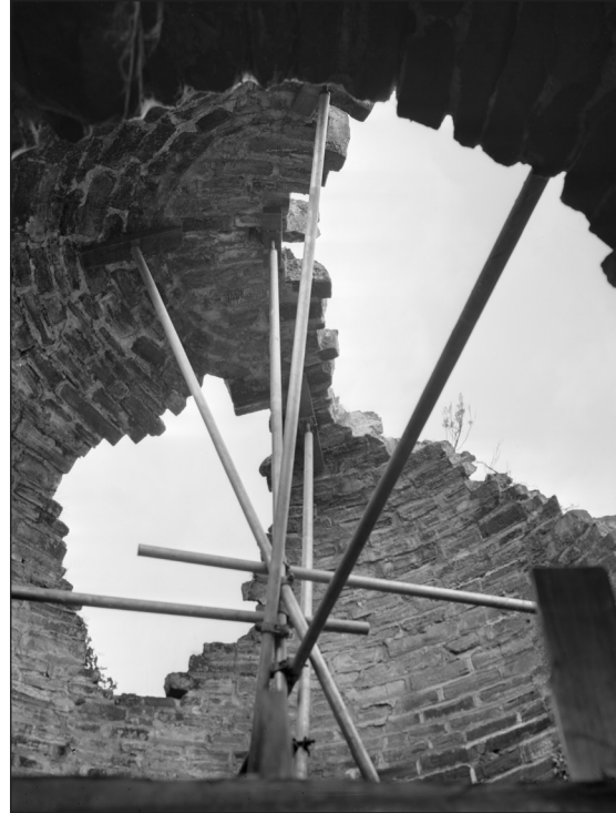
Fig. 55 The roof of the bath room, shored up in November 1956 after partial collapse (p_a04542_006 Historic England Archive)
