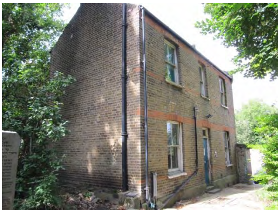
Caretaker's house and view to street door; water penetrarion, rotten timbers, broken windows etc. Path on right view may have burials under.
