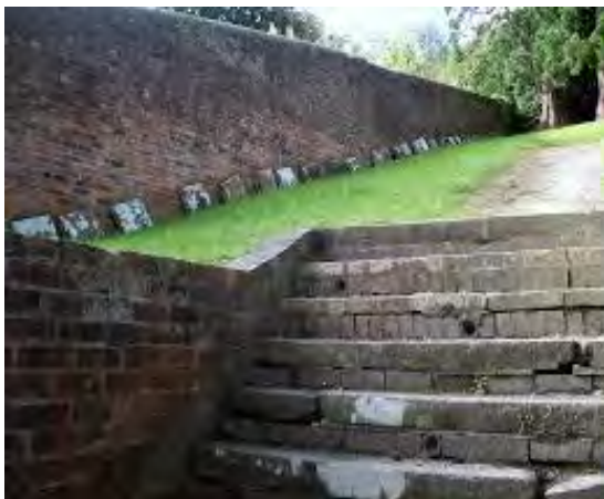
Steps to Ground showing condition
