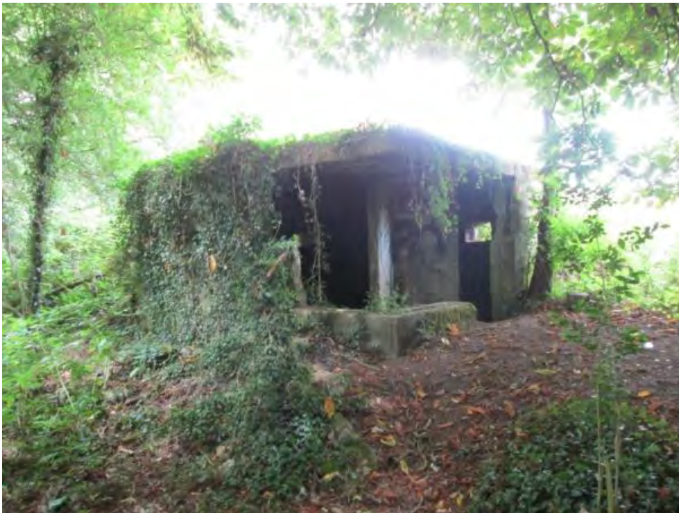
Pillbox at north boundary, damaged.
