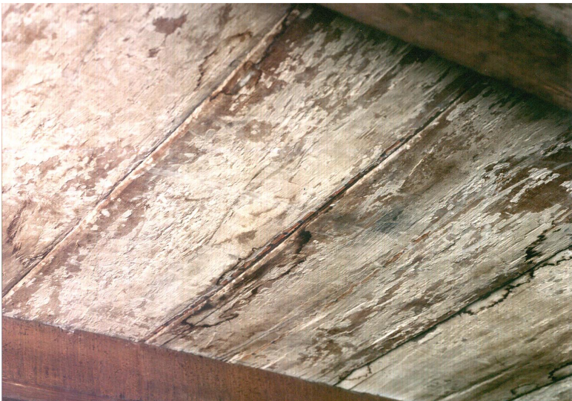
Figure 19: Photo of underside of shelf or canopy boards, Pyx Chamber, showing painted decoration (P Payne)
