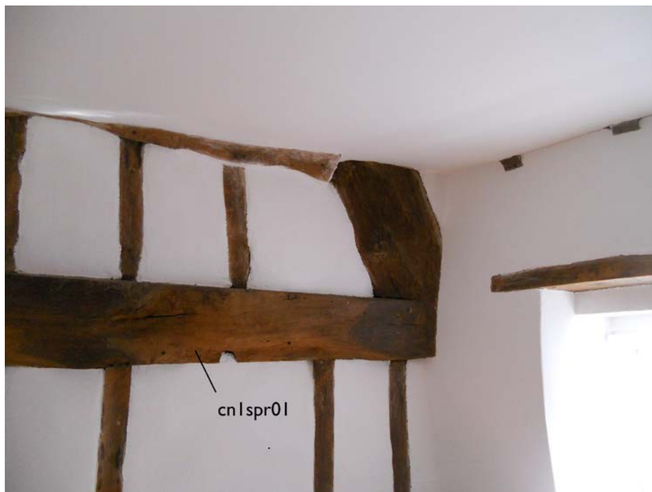
Figure 4: Photograph showing the tiebeam of the north truss sampled for dendrochronology (photograph Martin Bridge)
