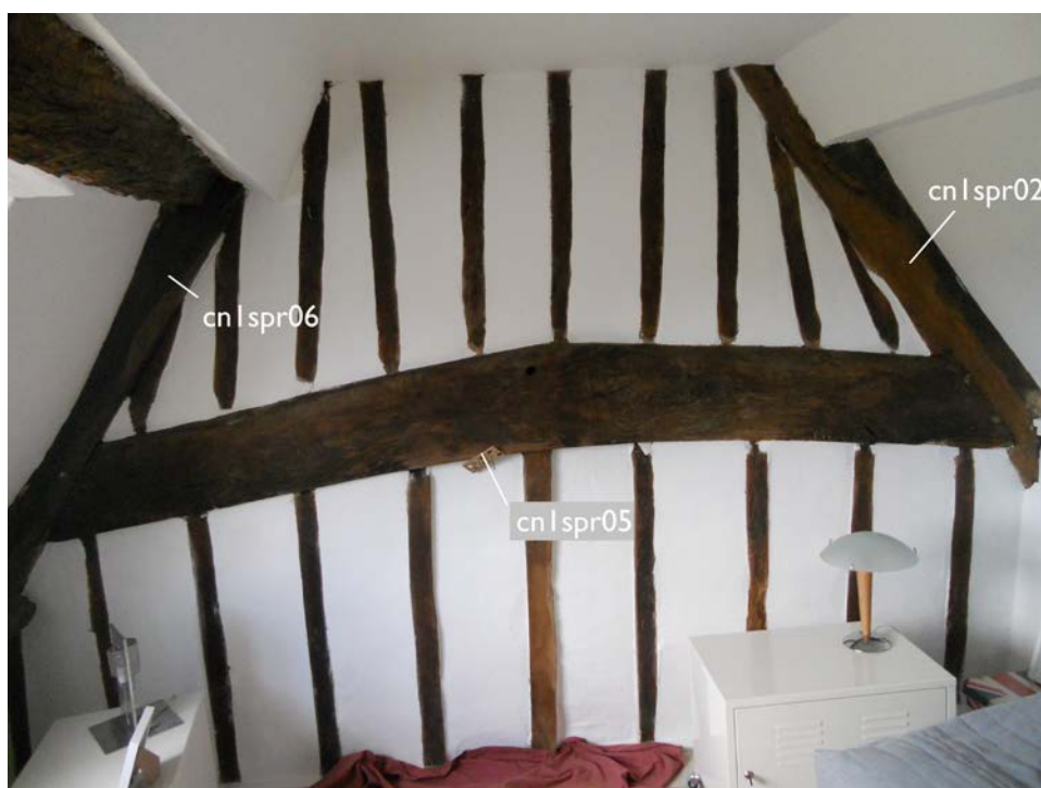
Figure 5: Photograph showing the north truss at first-floor level, indicating timbers sampled for dendrochronology (photograph Martin Bridge)
