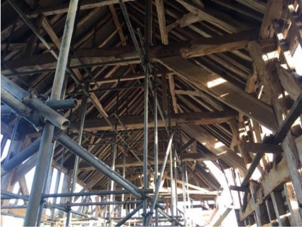
Figure 3: The roof over the main body of the barn, photograph taken from the west (photograph Alison Arnold)
