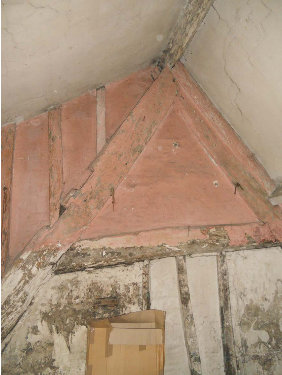
Figure 4: Photograph (looking east) of the upper part of the truss at the truncated west end of the east-west range (photo Martin Bridge)
