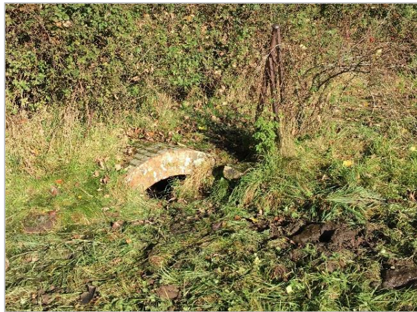
Figure 11 Catchwork water meadow feature comprising a bridge and culvert at Bagmore Farm, near Silton
