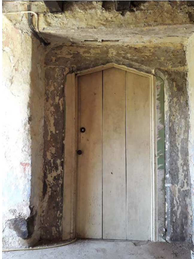
Figure 7: The doorway from the cross-passage into the hall, photograph taken from the east (Alison Arnold)
