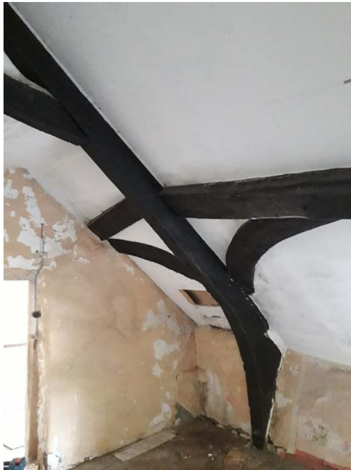
Figure 4: Truss 2, with purlins and surviving windbraces, photograph taken from the north-west (Alison Arnold)
