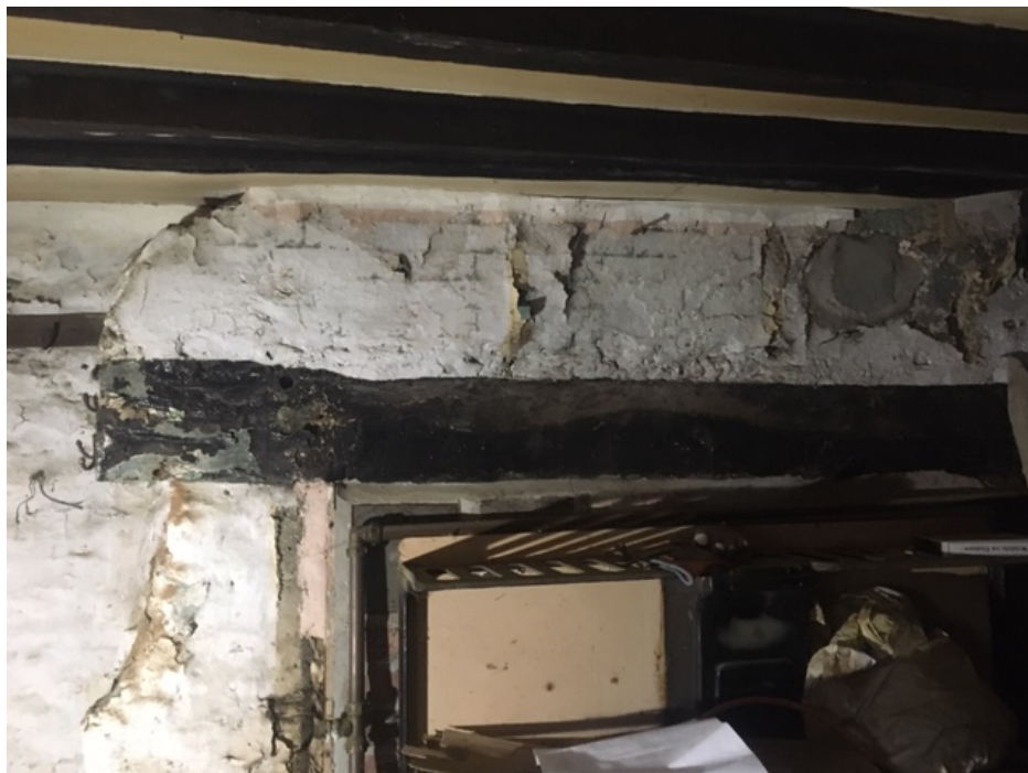
Figure 8: High end (present kitchen) fireplace bressummer, photograph taken from the east (Alison Arnold)
