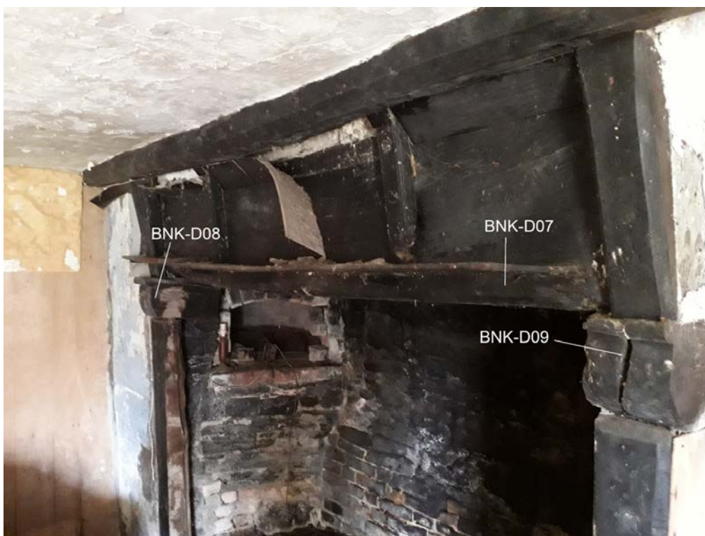
Figure 6: Hall (present living room) fireplace, showing the location of sampled timbers BNK-D07–09, photograph taken from the south-west (Alison Arnold)
