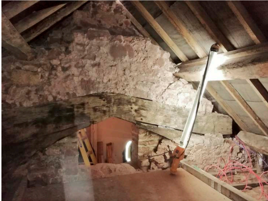
Figure 2: View of the south remnant medieval truss in the south roof, looking north (photograph Martin Bridge)
