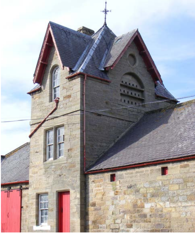
At East Allerdean (early 19th century), the arched and gabled entry to the main yard breaks the line of the range at its centre point. The three tiers of pigeon holes sit in a recessed area under the eaves. Photo © Jen Deadman
