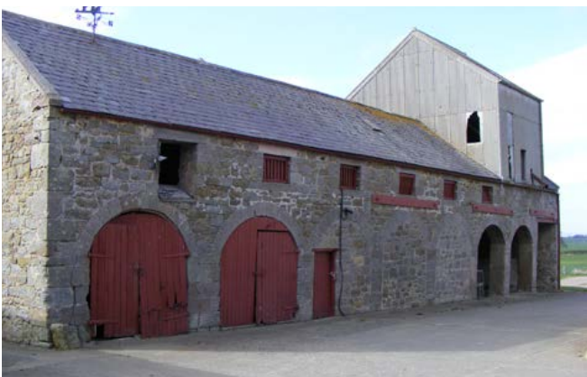
Granaries A large, eight-bay cart shed with a granary over. A 20th-century corn drier with an auger, to lift corn to the granary, now straddles the roof of the granary. Photos © Jen Deadman
