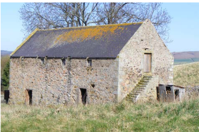
Defensible farmsteads. The remains of the former bastle at Akeld, near Wooler, is possibly of 16th-century origin. It is large for a bastle, and possibly served as a communal 'stonghouse' at the head of the village street which, by around 1800, had been swept away by the present farm hamlet. Of the original building, only the ground floor remains, the rest having been rebuilt in the 18th century. It is not directly associated with a farmstead complex, although the former Manor House stands close by. Oval-shaped earthworks in the vicinity of the building are suggestive of an enclosure and/or foundations of early farm buildings. In the roof of the barrel vault to the ground floor is a small hole which would have allowed access to the upper floors by a ladder. In times of trouble, stock and stores would be secured in the room, the door bolted and barred from the inside and the ladder withdrawn. In more recent times the ground floor has been used as a cattle shelter and the first floor as a granary.
