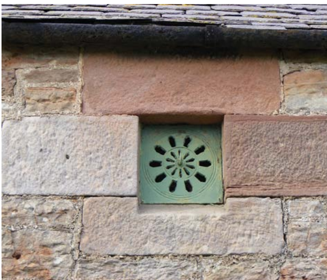
Detail showing cast-iron ventilator and the quality of the stone masonry. Photo © Jen Deadman
