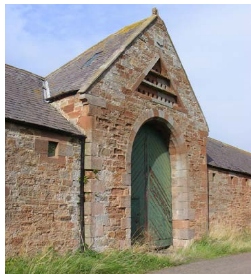
Detail showing doveholes over the entrance to the covered yards of 1879. Photo © Jen Deadman
