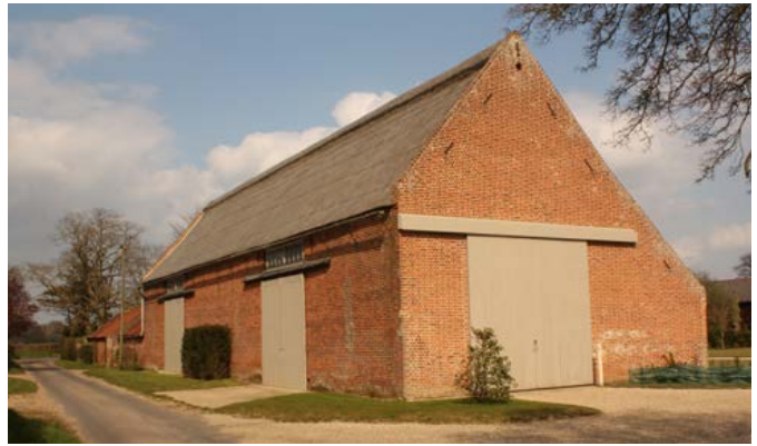
This large 19th-century barn of six or seven bays in length was built with an aisle to the rear, possibly providing additional storage area within the barn rather than animal housing. Aisled barns are extremely rare in this area, although they are a distinctive feature of much of East Anglia. Photo © Bob Edwards
