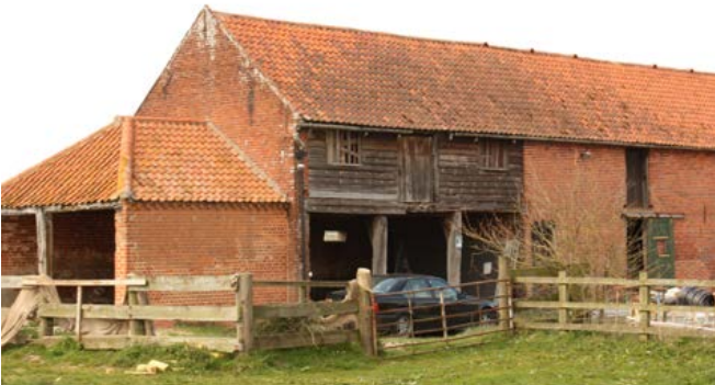
Granaries are not a common feature of farmsteads in this area. Where found, they are usually of 19th-century date and located over a cart shed. This example forms part of a long range with stables which have a hay loft over. An additional two bays for carts and equipment have been added against the gable wall of the range. Photo © Bob Edwards
