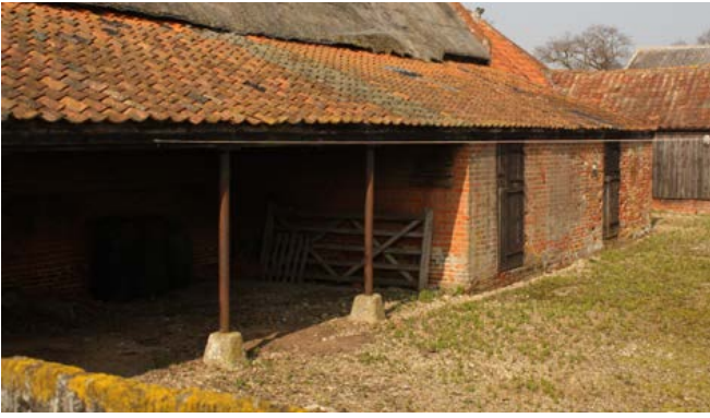
Shelter sheds could also be built against the side of a barn. Here, a three-bay shelter shed is accompanied by two loose boxes for cattle. Photo © Bob Edwards.
