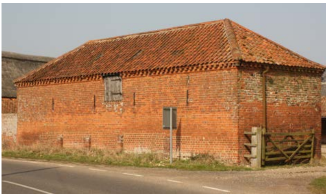
Although there was very limited arable on the marshland the farmsteads surrounding the marshes had access to the fertile arable land. Therefore most farms had stables for the working horses. Many date from the 18th century and are two-storey buildings with a hayloft above stables. Photo © Bob Edwards.
