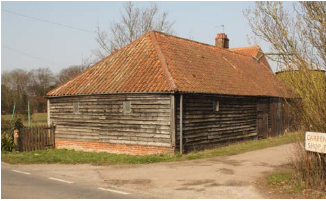
Workshops A timber-framed, single-storey shed that may have served as a workshop. Photo © Bob Edwards.
