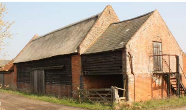
Granaries are uncommon in this area. Where found, they are usually located about the cart shed and date from the 19th century. This example has been built against the gable of an earlier barn, the cart shed typically facing away from the yard. Photo © Bob Edwards.
