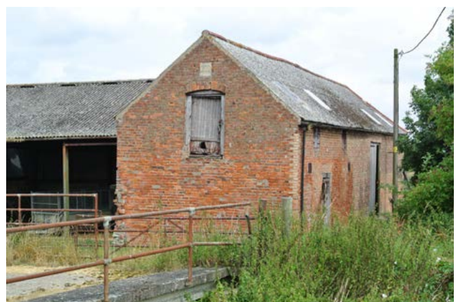
Neslam Fen Farm, a small field barn with modern cattle sheds attached. Although in some disrepair, the building is still in agricultural use. Photo © Locus Consultants
