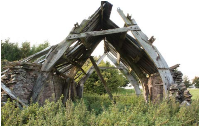
A small, three-bay, cruck-framed cow house located within the foot hills of the Black Mountains. Examples such as this are very rare surviving examples of building types and traditions that were largely swept away in the 18th and 19th centuries. Photo © Bob Edwards
