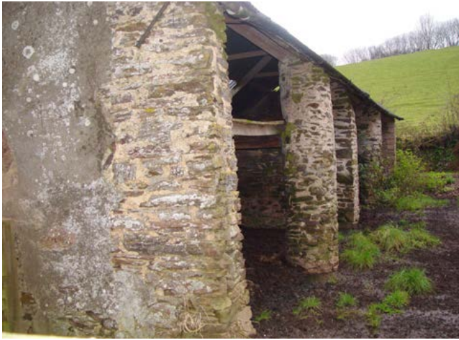
Stone piers are found commonly to shelter sheds but those to lincays occur occasionally, and more so towards the south and eastern fringe. This linhay has lost much of its upper floor. Photo © Philip White
