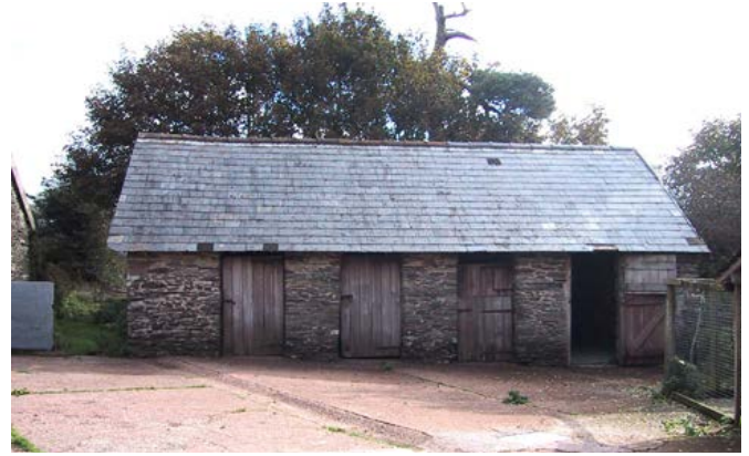
Another pigsty, typical of the south-west, with low eaves and no external feeders or runs. Photo © Philip White
