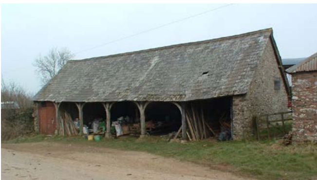
An open-fronted cart shed, with one closed, lockable bay, typically facing onto a track. It caters for carts, field implements and more valuable equipment. Photo © Philip White
