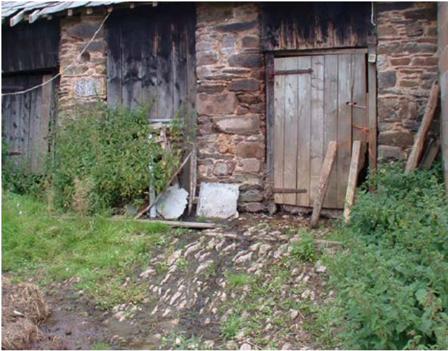
Stone cobbling is a significant feature of farmyards. It informs us about animal buildings, housing arrangements and movement in the yards. Photo © Philip White
