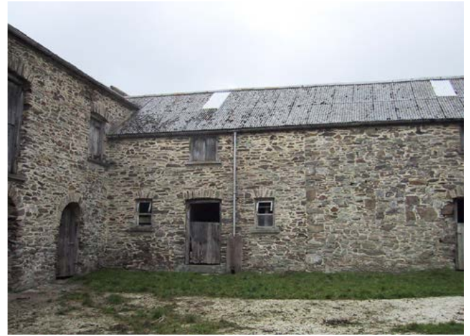
The vertical joint in this construction is indicative of a later phase of extension to the original work. The position of the larger, former quoin stones shows the earlier work. Many buildings were extended to provide additional housing for cattle. Photo © Philip White
