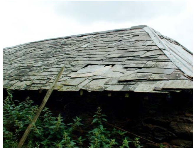
Original Exmoor slate is now a rare find. This old, failing roof, covered in a mix of mostly local slates, has been fixed without battens, directly to rafters, akin to a form of rag work. Photo © Philip White
