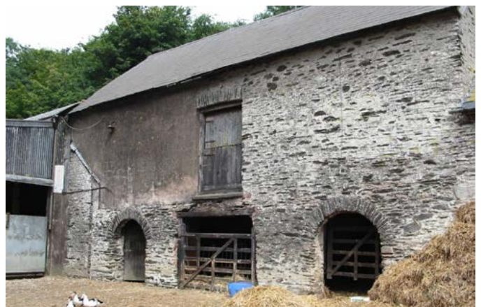
A typical medium-size bank barn in a courtyard layout. The external lime plastering still shows evidence of the trowel marks found on many Exmoor buildings. Photo © Philip White
