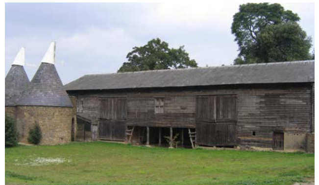
A large, mid-19th-century multifunctional barn with two threshing bays. In between there is a shelter shed for cattle and to the right a stable. The left end possibly served as the stowage attached to the hop drying kilns. Photo © Historic England
