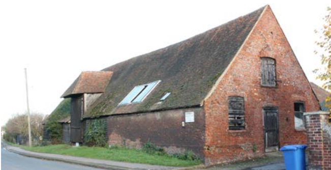
One of two large barns on a high-status farmstead, this barn has been partly rebuilt in brick and incorporates stabling with a hayloft above. Photo © Bob Edwards
