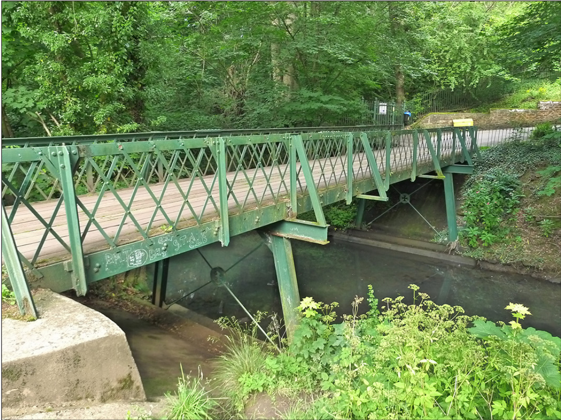
Fig 20. The pony truss bridge over the River Gaunless in Bishop Auckland Cemetery. (© Historic England/Marcus Jecock)
