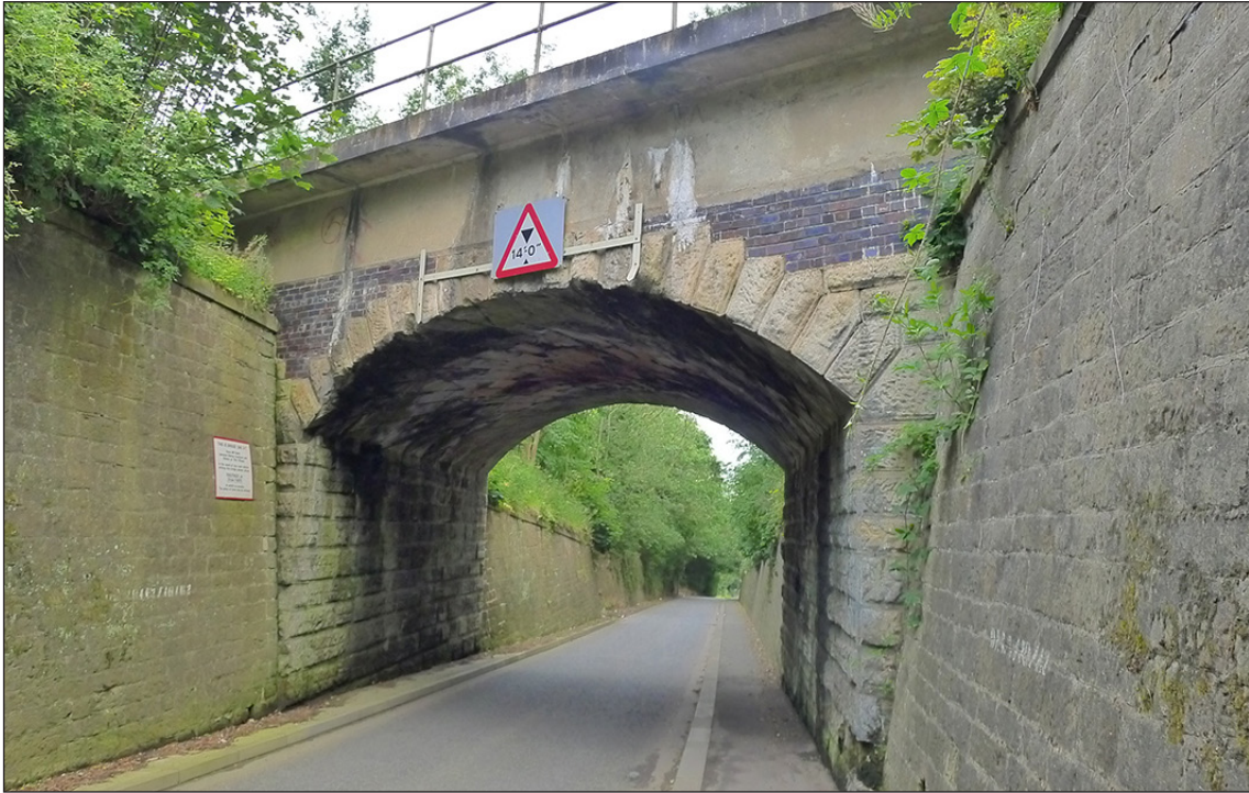
Fig 59. The north-east (uphill) elevation of railway underbridge DAE2/7 (Bone Mill Bank). Note the brick repair to the spandrel and the later concrete parapet. (© Historic England/Marcus Jecock)
