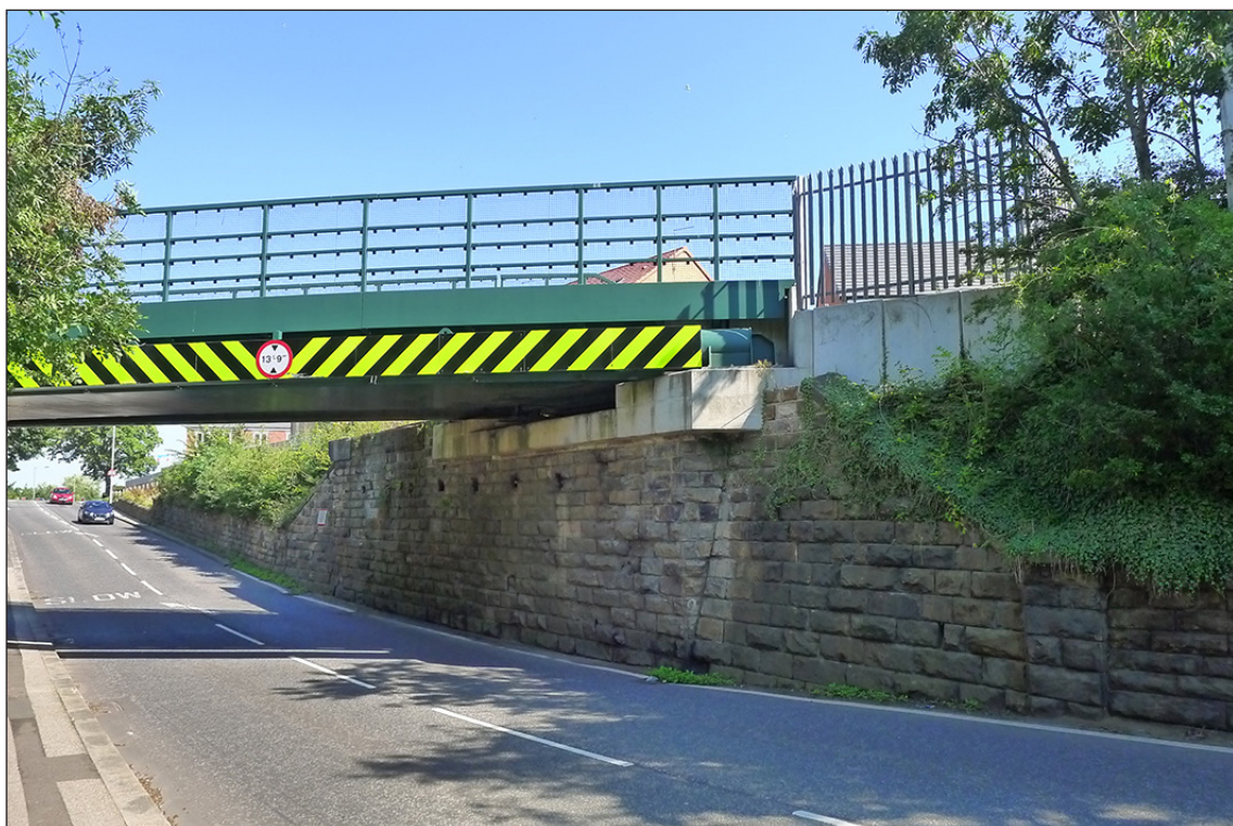
Fig 66. The south elevation of railway underbridge DAE2/9 (South Church Lane). Note the modern concrete bearing block which has replaced the topmost courses of stonework in the abutments. (© Historic England/Marcus Jecock)
