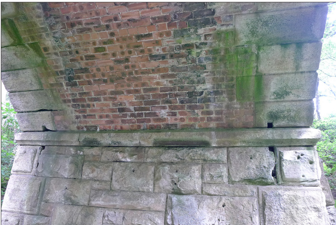
Fig 47. Detail of abutment face and brick arch barrel of railway accommodation bridge BIF/12, showing impost band plus the varied finishes applied to the stonework. (© Historic England/Marcus Jecock)
