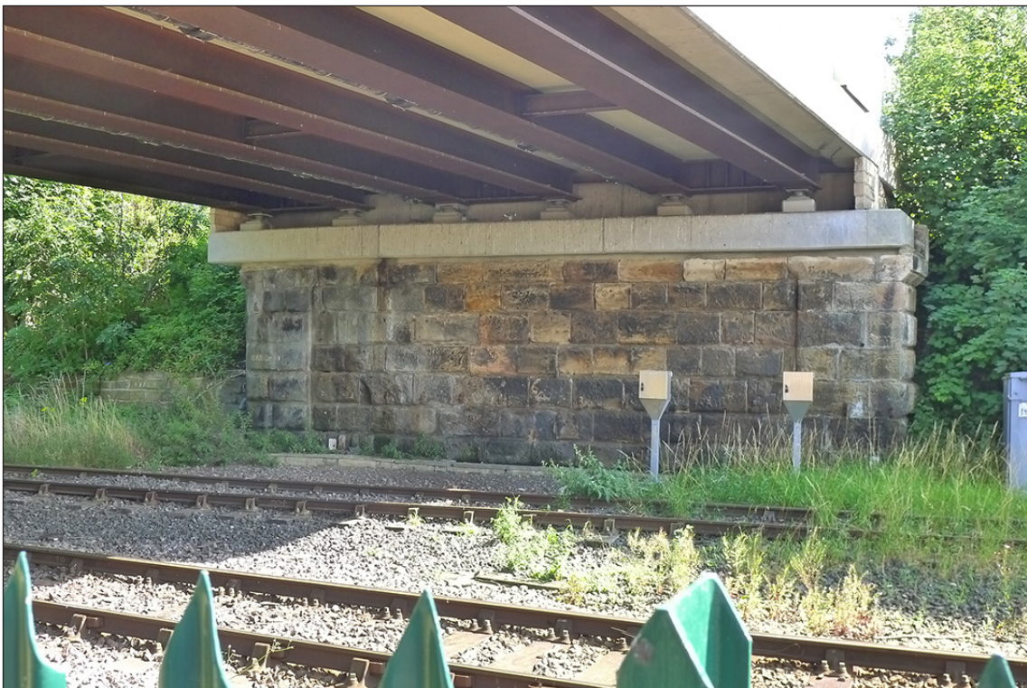
Fig 69. The south abutment of railway overbridge DAE2/10 (Cockton Hill Road). Note the ends of the abutment break forward slightly and are surmounted by large ashlar blocks that corbel out on both sides, suggesting they initially comprised free-standing piers. (© Historic England/Marcus Jecock)
