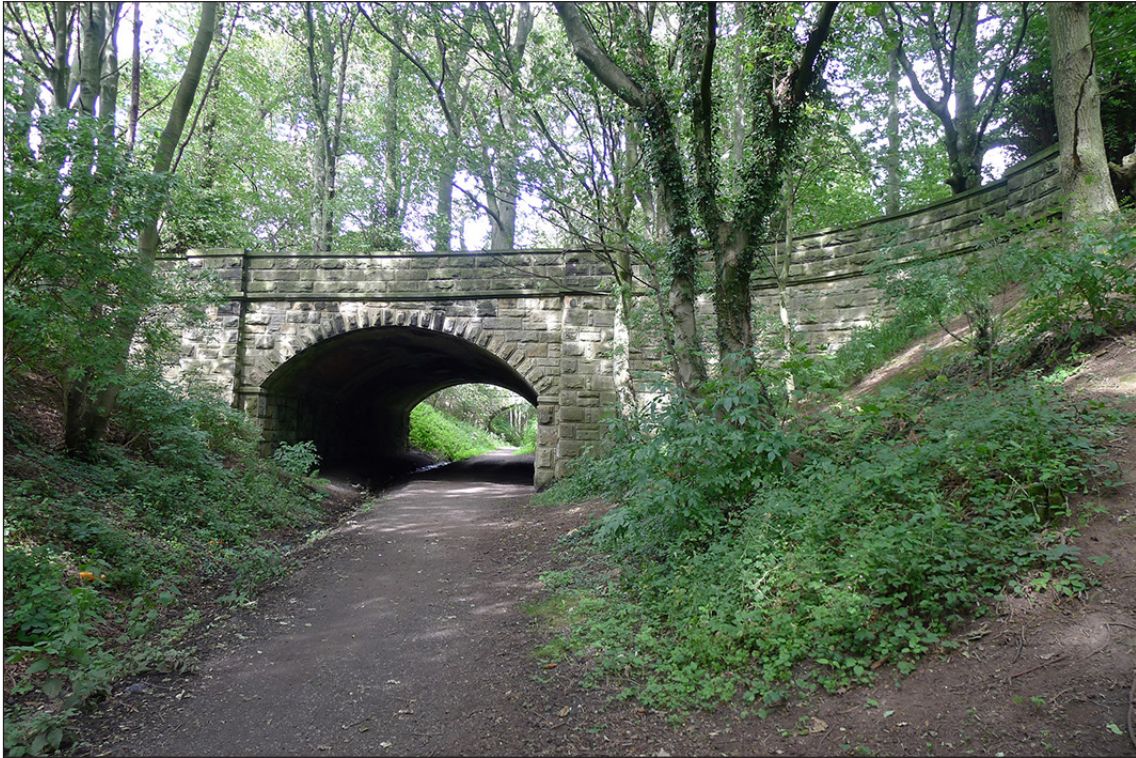
Fig 43. The south elevation of railway accommodation bridge BIF/11 ('Bishop's Bridge'). Note the great width (or length) of the arch barrel. (© Historic England/Marcus Jecock)
