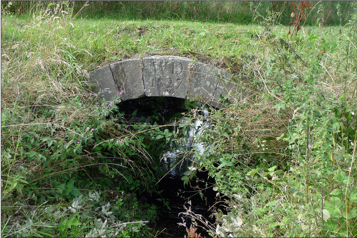
Fig 90. The upstream arch ring and inscribed keystone to Bishop Van Mildert's drive bridge over the Coundon Burn in Auckland Park. (© Historic England/Marcus Jecock)
