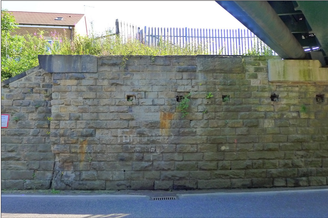
Fig 67. The north end of the east abutment of railway underbridge DAE2/9 (South Church Lane). Note the disused stone bearing blocks towards the centre and at the end of the abutment, and the modern tie rods and anchor plates added to stabilise the structure. (© Historic England/Marcus Jecock)
