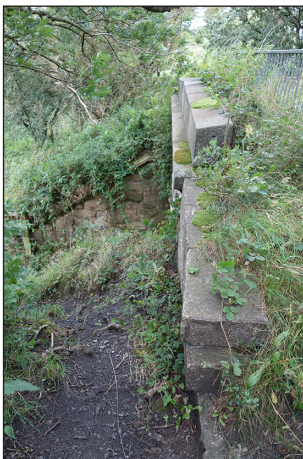
Fig 41. Detail of dislodged/missing stones in the eastern parapet of railway accommodation bridge BIF/10. (© Historic England/Rebecca Pullen)
