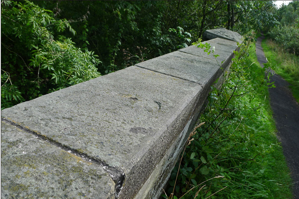
Fig 38. The (?replacement) western parapet of railway accommodation bridge BIF/9. (© Historic England/Marcus Jecock)
