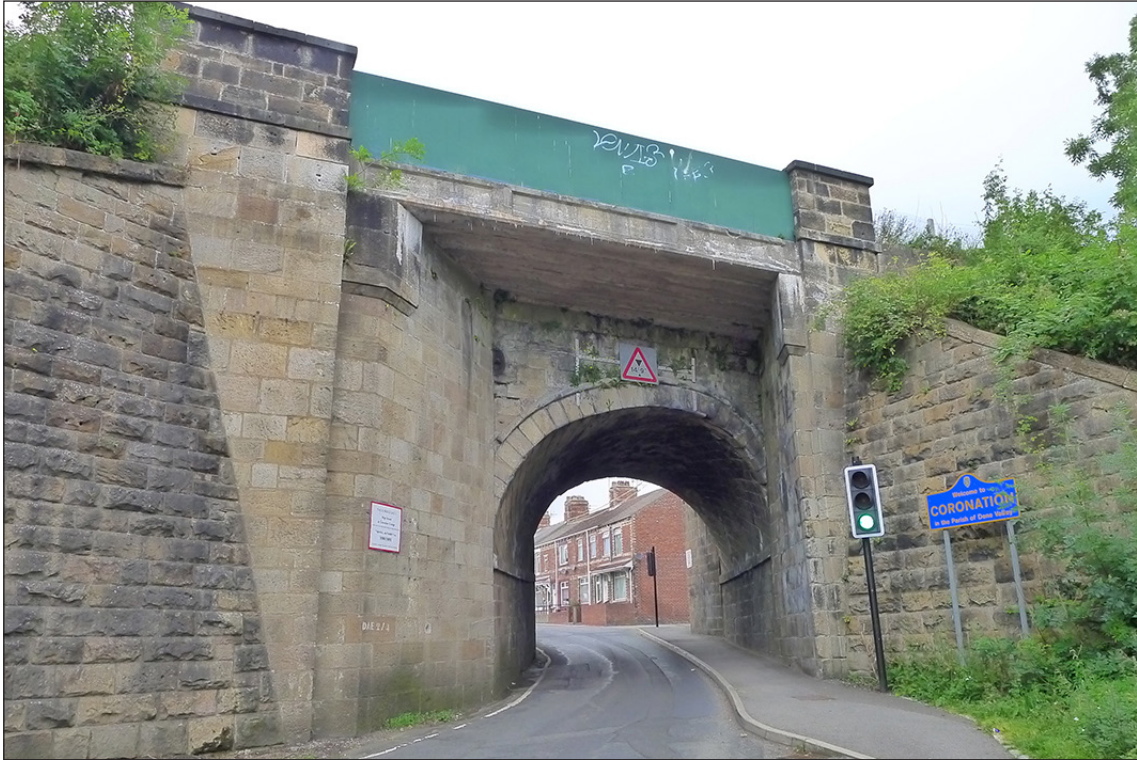
Fig 52. The eastern elevation of railway underbridge DAE2/4 (High St, Coundon Grange), showing the original skew arch and one half of the later widening. (© Historic England/Marcus Jecock)
