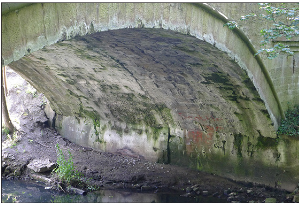
Fig 15. The construction joint visible in the barrel of Gaunless Bridge. (© Historic England/Marcus Jecock)
