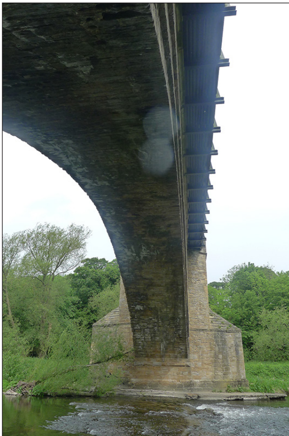
Fig 8. The underside of the southern arch and the central pier of Newton Cap Bridge seen from the south. (© Historic England/Marcus Jecock)
