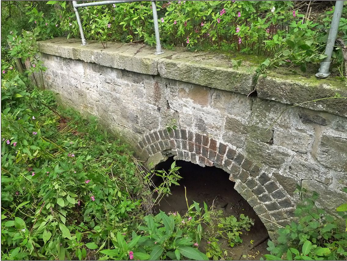
Fig 56. The southern headwall of culvert DAE2/5 taking Dene Beck under what was originally the Bishop Auckland & Weardale Railway, now the Darlington to Bishop Auckland line. (© Historic England/Marcus Jecock)
