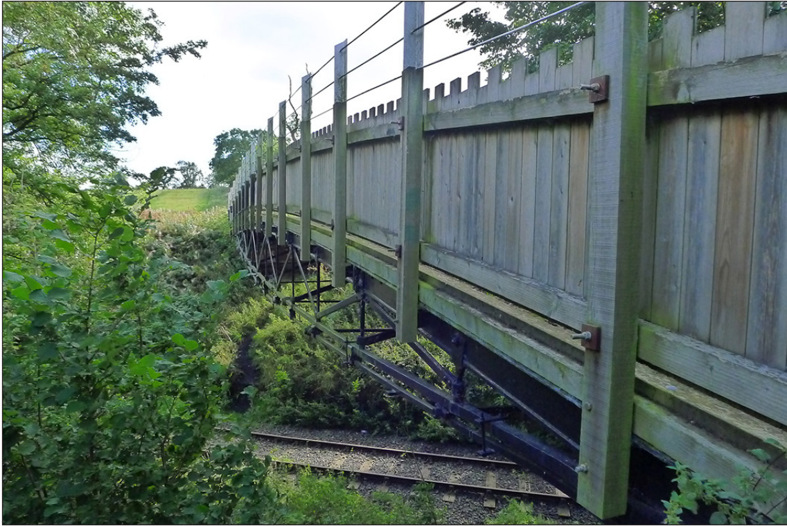
Fig 74. The eastern elevation of railway accommodation overbridge DAE2/12 (lenticular truss), looking south. (© Historic England/Marcus Jecock)
