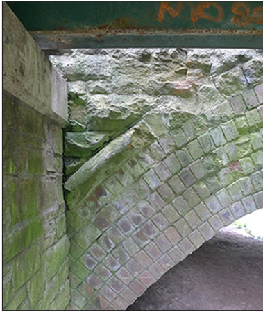
Fig 24. The hacked archivolt close to the eastern springing of the phase-2 B6282 bridge at South Church. (© Historic England/Marcus Jecock)
