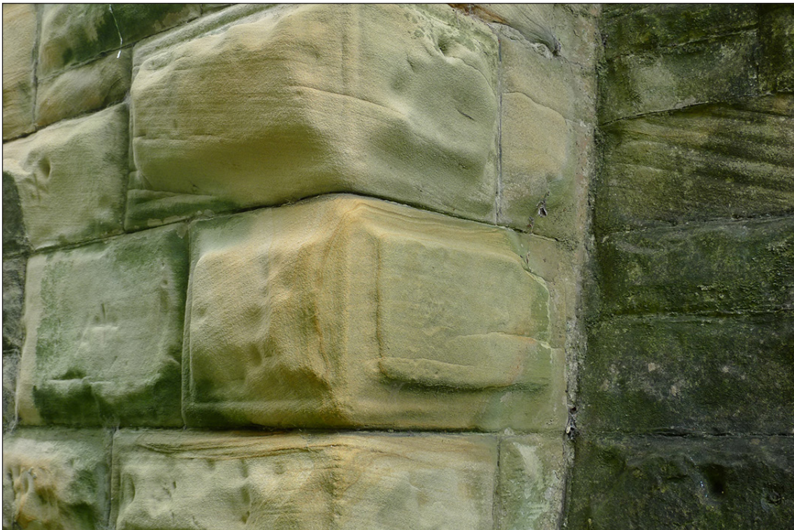
Fig 36. Detail of the weathered stonework on the abutment of railway accommodation bridge BIF/9. (© Historic England/Marcus Jecock)
