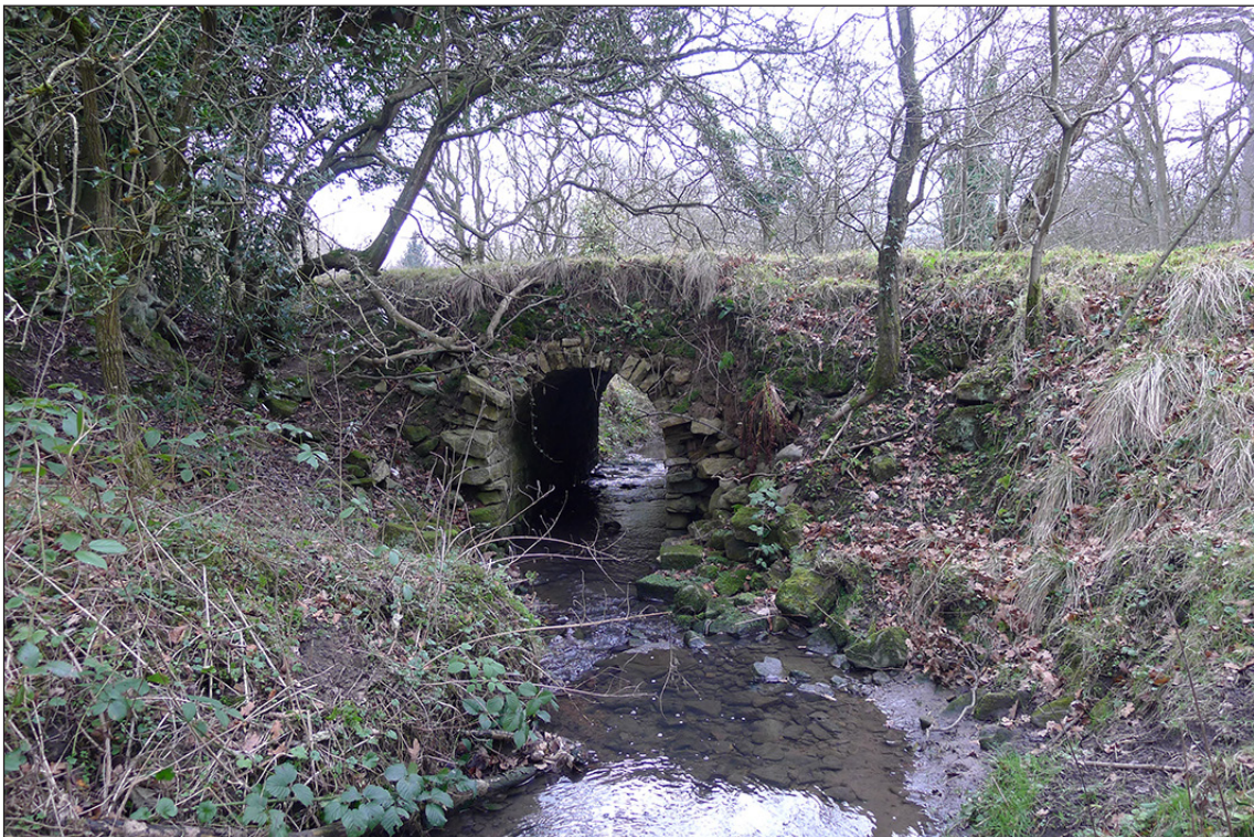
Fig 89. The collapsed, upstream (eastern) arch ring and headwall of 'footbridge no. 3' across the Coundon Burn in Auckland Park. (© Historic England/Marcus Jecock)
