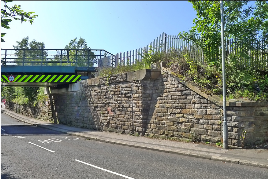
Fig 65. The north elevation of railway underbridge DAE2/9 (South Church Lane). (© Historic England/Marcus Jecock)
