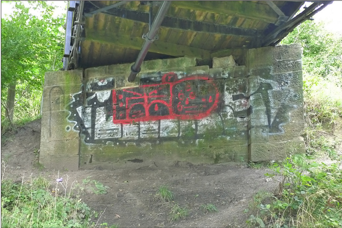
Fig 76. The face of the north abutment of railway accommodation overbridge DAE2/12 (lenticular truss). (© Historic England/Marcus Jecock)
