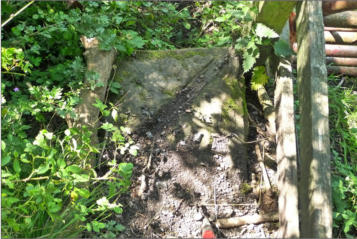
Fig 42. Detail of one of the end pier caps to the retaining walls of railway accommodation bridge BIF/10, showing the 'half-saltire' channelling. (© Historic England/Marcus Jecock)
