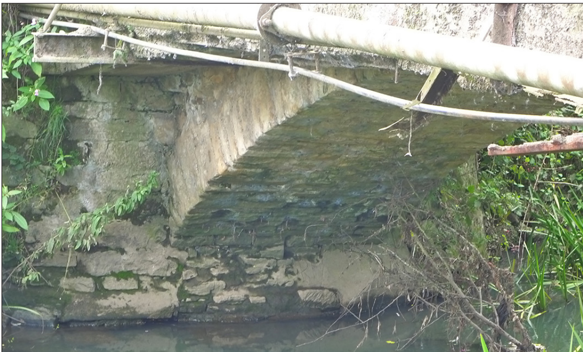
Fig 27. Detail of the southern abutment and arch of the 'Deanery' packhorse bridge across the River Gaunless at South Church. (© Historic England/Marcus Jecock)
