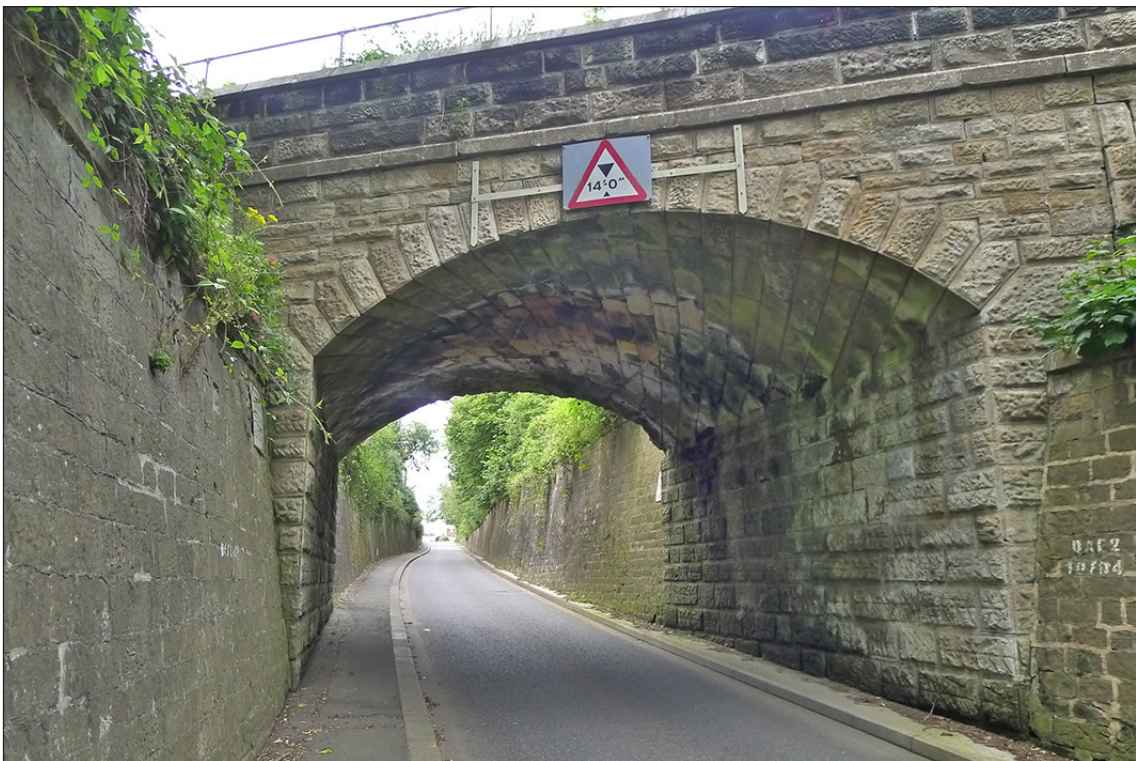
Fig 62. The south-western (downhill) elevation of railway underbridge DAE2/7 (Bone Mill Bank). (© Historic England/Marcus Jecock)
