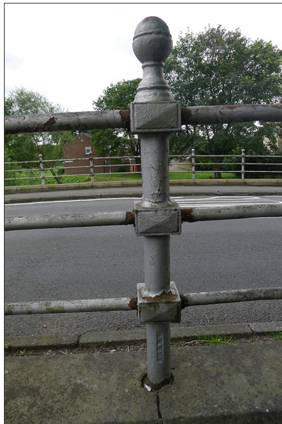
Fig 25. Detail of the Inter-War railings to the B6282 bridge over the River Gaunless at South Church. (© Historic England/Marcus Jecock)
