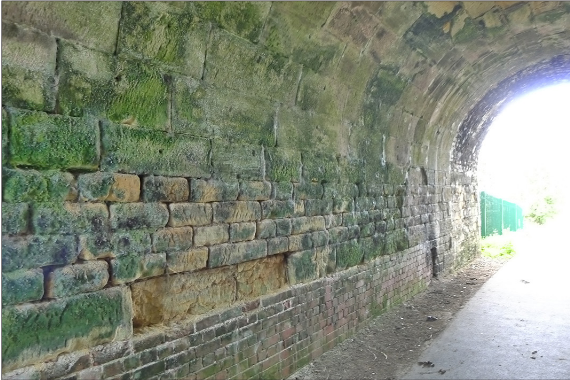
Fig 57. The southern face of the phase-1, abutment of railway accommodation underbridge DAE2/6 ('Shepherds'). Note the repeating rhythm of the original stonework: four narrow courses followed by one course of larger stones, all now deteriorating and heavily patched in brick. The stone arch barrel contrasts with the brick arch barrel of the phase-2 western extension which can just be made out at right of frame. (© Historic England/Marcus Jecock)
