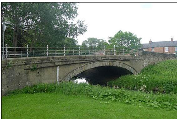
Fig 22. The southern (upstream) elevation of the phase-1 B6282 bridge over the River Gaunless at South Church (© Historic England/Marcus Jecock)
