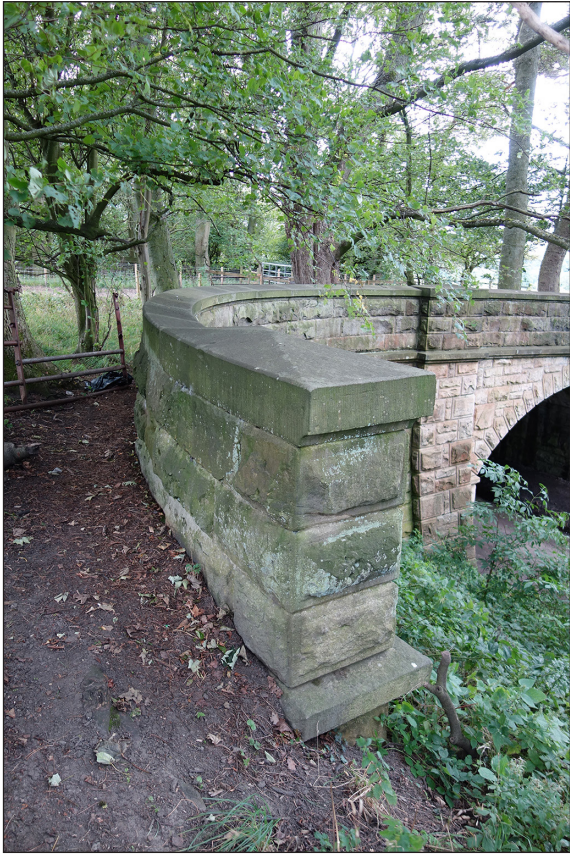
Fig 45. Detail of parapet and curving wing wall to railway accommodation bridge BIF/11 ('Bishop's Bridge'). (© Historic England/Rebecca Pullen)
