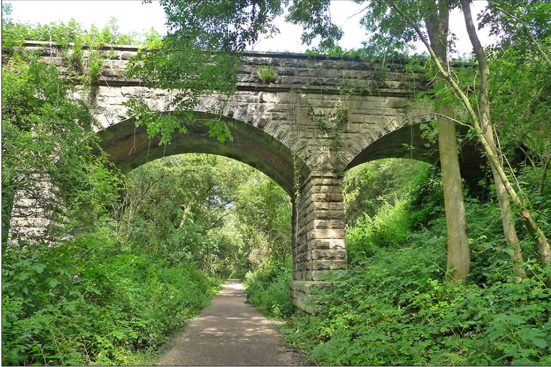
Fig 28. The south-western elevation of railway accommodation bridge BIF/5, showing the central and eastern spans. (© Historic England/Marcus Jecock)
