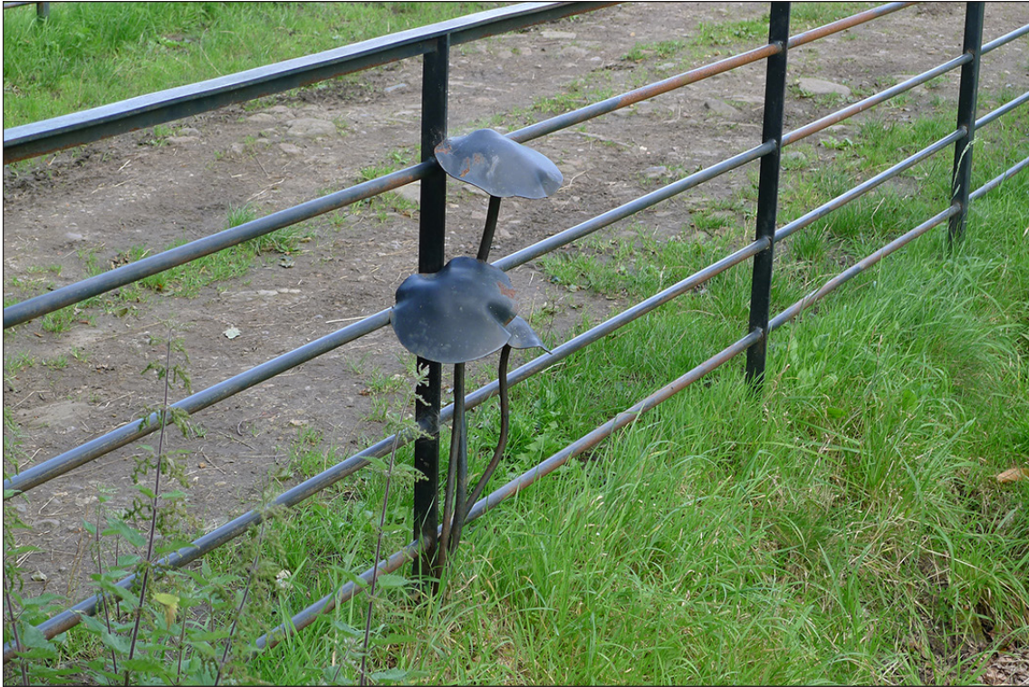
Fig 82. Detail of the modern railings to 'Bishop Trevor's' culvert for the Coundon Burn in Auckland Park. (© Historic England/Marcus Jecock)
