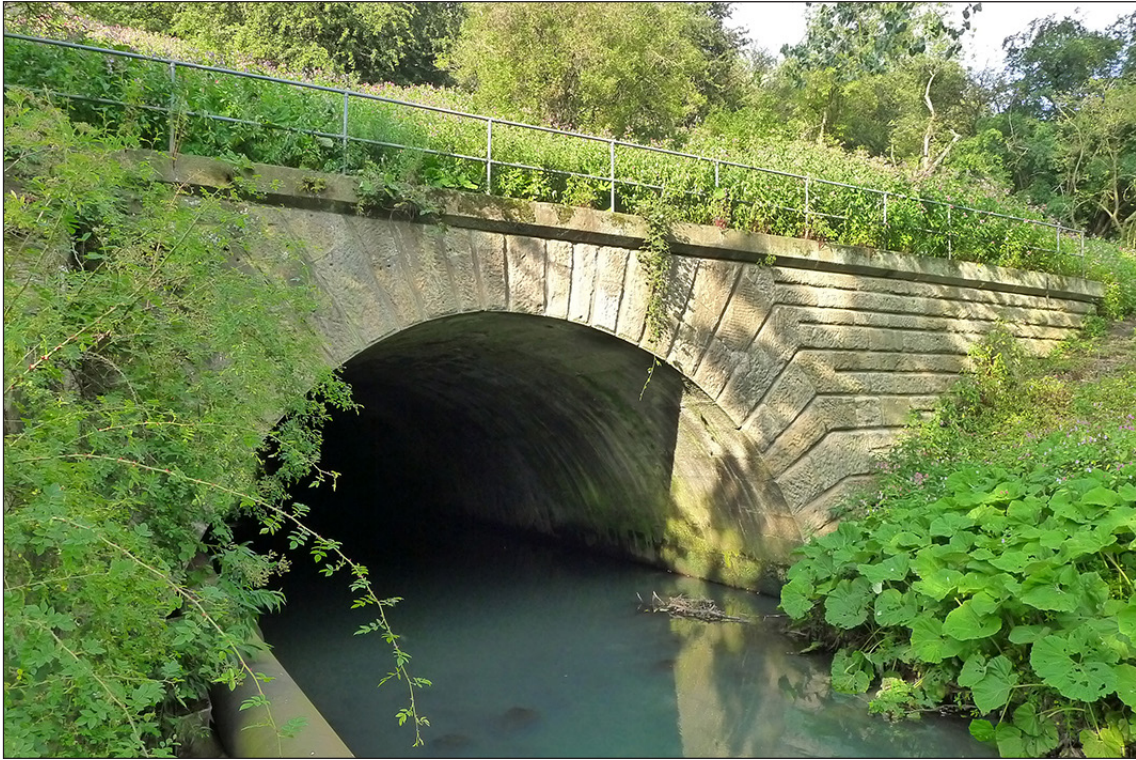
Fig 63. The southern portal of railway bridge DAE2/8 over the River Gaunless. (© Historic England/Marcus Jecock)
