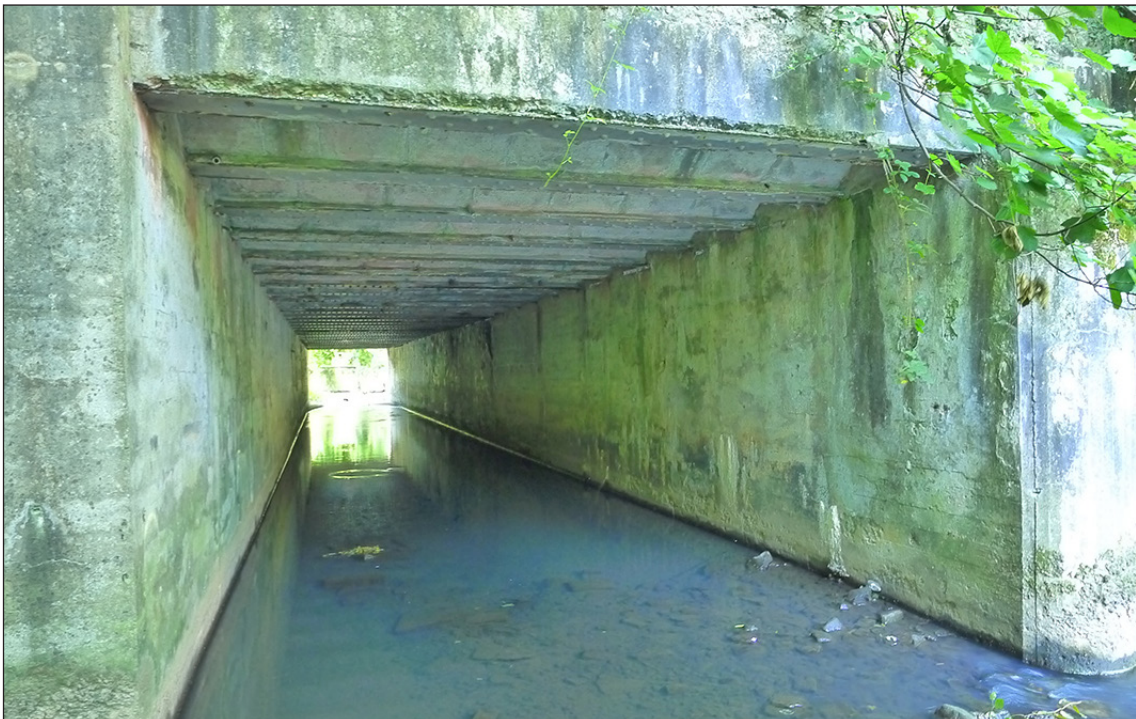
Fig 14. The eastern of the two box conduits of the bridge carrying Durham Road across the River Gaunless., seen from the north. The central spine wall with its bullnose cutwater is at right of frame. Note the soffit formed from steel joists and concrete jack arches. (© Historic England/Marcus Jecock)
