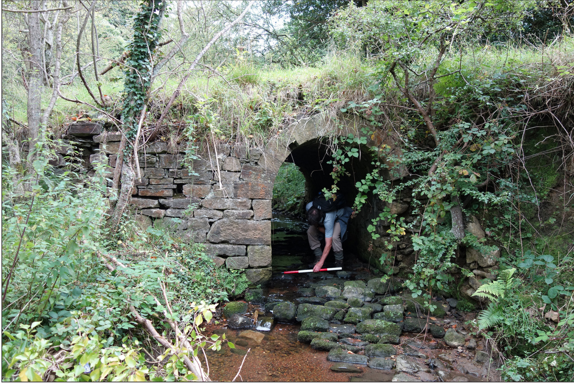
Fig 88. The downstream (western) headwall of 'footbridge no. 3' across the Coundon Burn in Auckland Park. (© Historic England/Rebecca Pullen)
