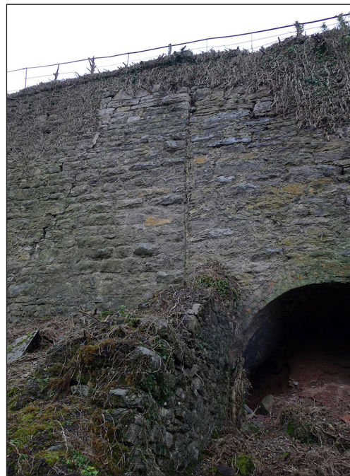
Fig 1. Construction join in northern elevation of the Bellmanpark kilns, showing that the western kiln (right of frame) is a later addition. (AF00393027 © Historic England / Marcus Jecock, 6 January 2016)
