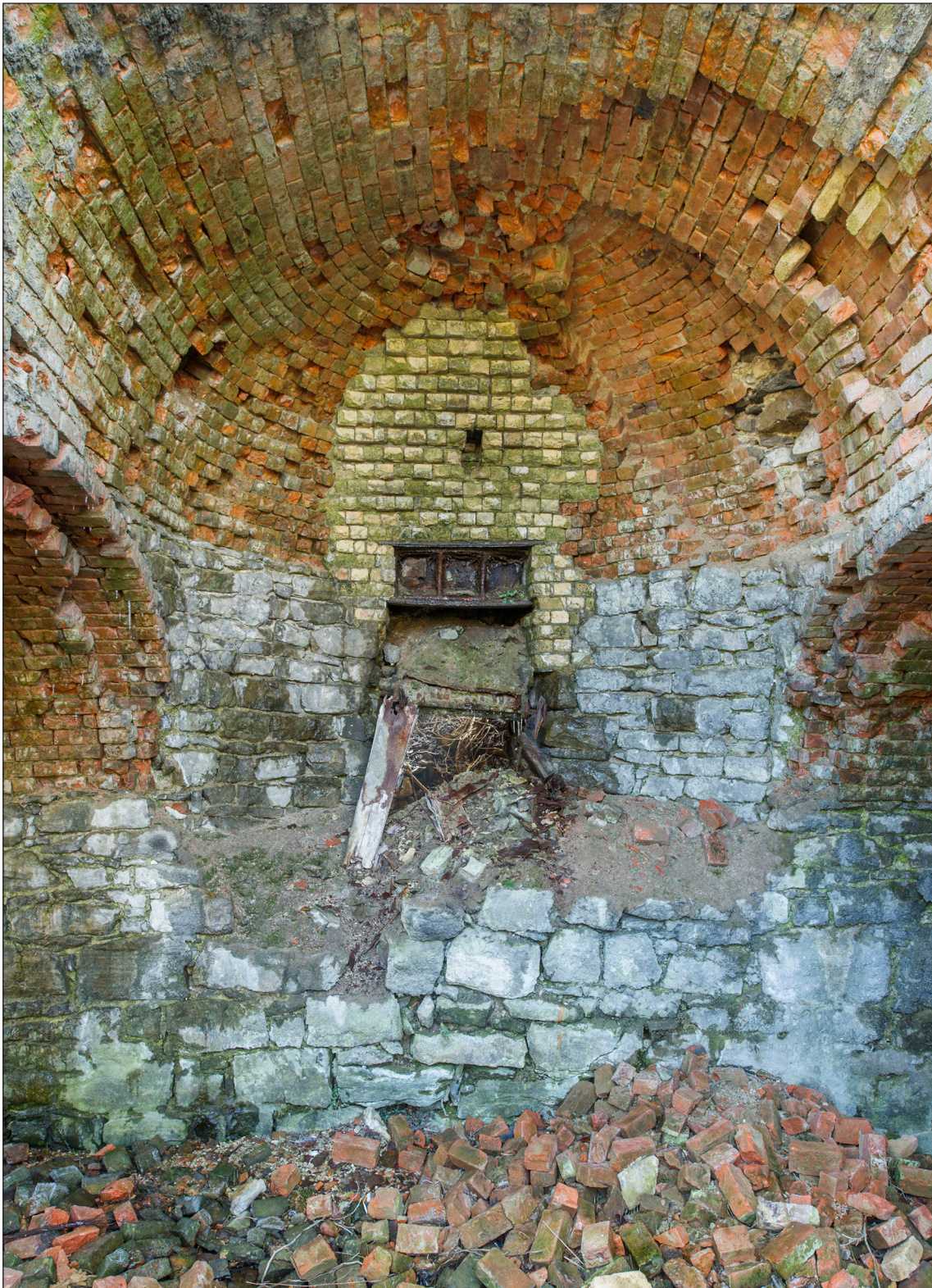
Fig 3. The collapsing northern draw arch to kiln 1, showing its intersection with the northern rail tunnel and the draw-hole furniture. (Photograph: DP169500 ©Historic England / Alun Bull, 24 February 2016).
