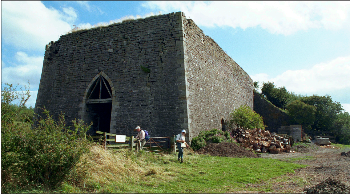
Fig 21. The Grade II*-listed Littlemill limekiln bank from the north, showing the entrance to the central rail passage. The top of what is probably an interconnecting cross passage can just be seen in the centre of the western (right-hand) wall. (© Mr Peter Oakley Clarke. Source Historic England, IoE No: 237036 Film No: 02000 Image: 31).
