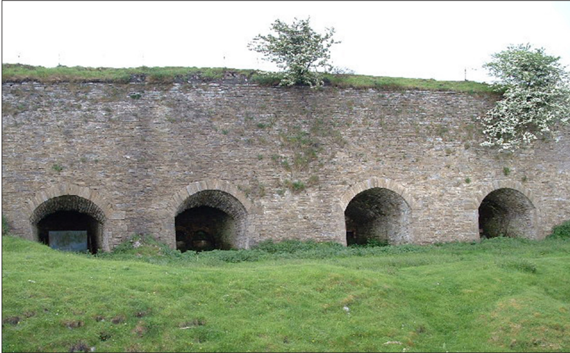
Fig 17. The scheduled Foresthead limekilns from the north-west. (© Malcolm Jones, https://www.cumbriacountyhistory.org.uk/farlam-1-ny5857-lime-kilns-forest-head-well-preservedjpg under Creative Commons Licence).
