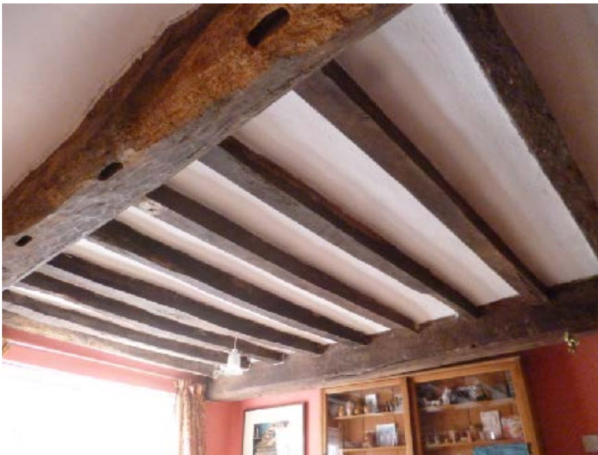
Figure 2a/b: Views, looking north-east, of the timbers to the ground-floor front room at Home Farm Cottage; wall-post and brace (top) and ceiling beams (bottom)(photographs Robert Howard)
