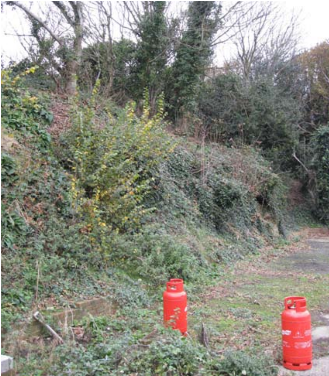
Plate 5. External rampart face exposed in Rocklands Caravan Park © Sarah Newsome
