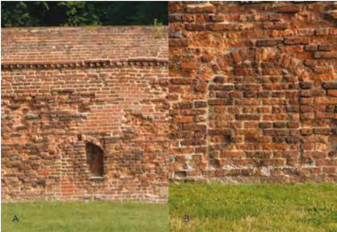
Figure 24: A - Section of the northern boundary wall showing one of the partially blocked bee boles, the dog-tooth string course and the ornamental coping. B - Detail of blocked bee bole.
