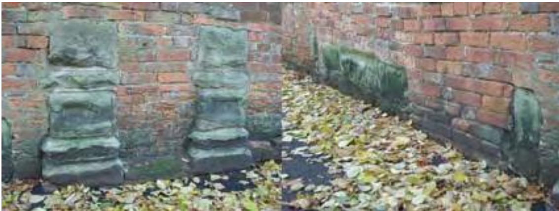
Figure 22: Masonry, probably reset, marking the possible position of gateways into the garden from Mount Walk.
