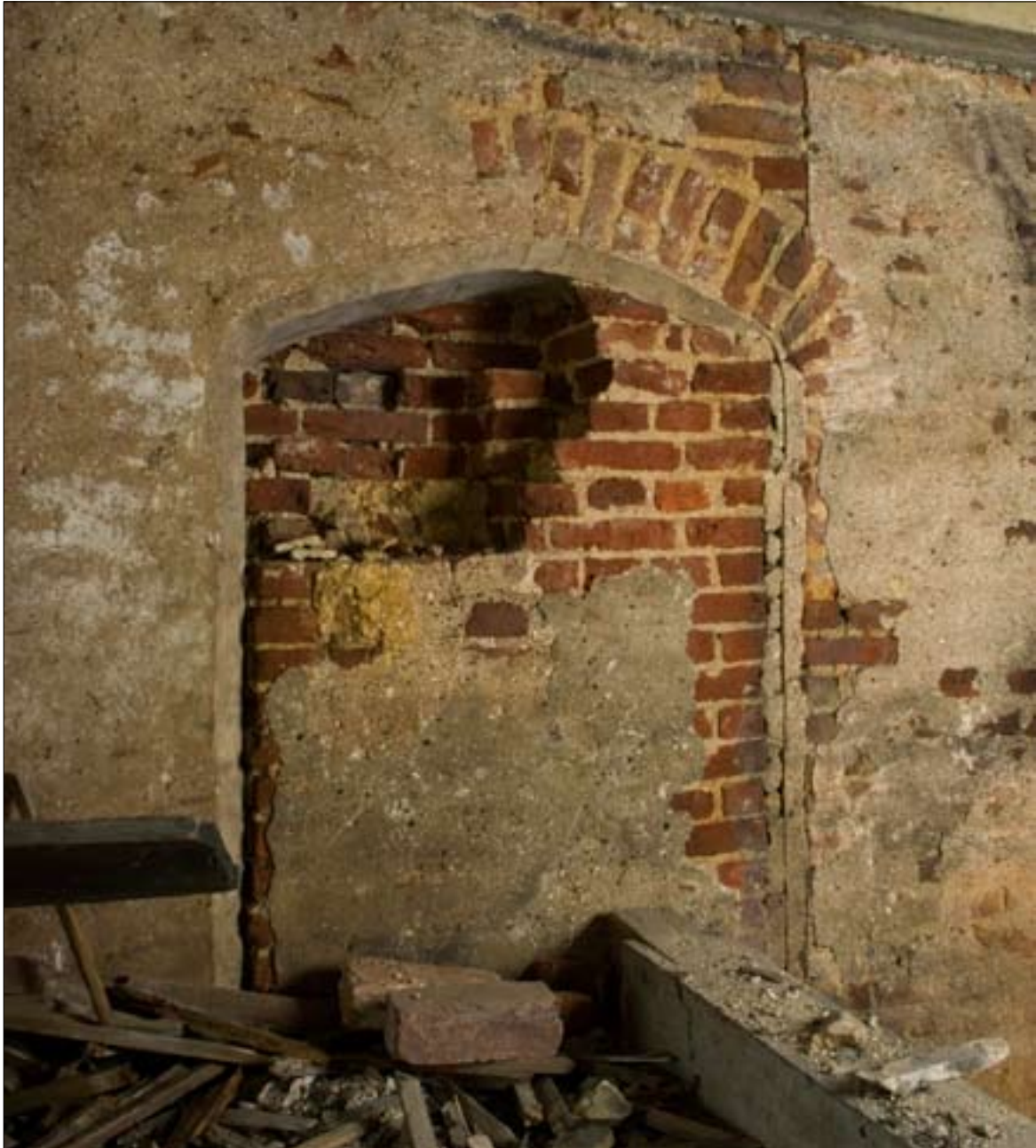
Fig. 17. The blocked doorway on the first floor in the west crosswing. © English Heritage DP029982
