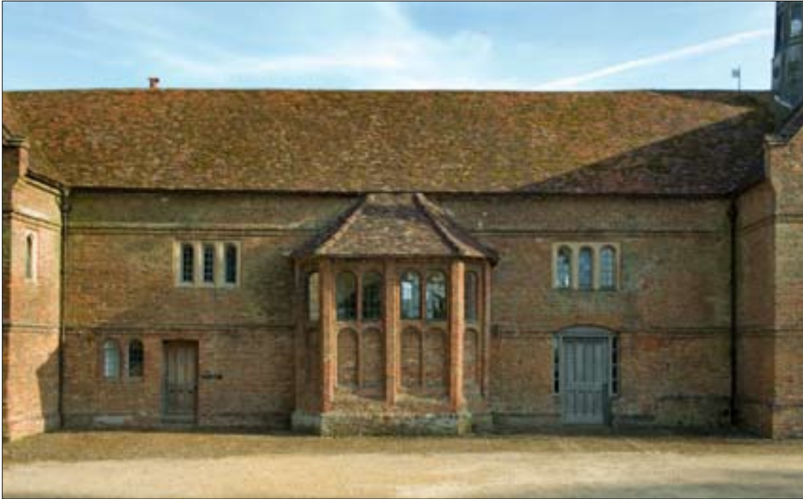
Fig. 36. The eastern section of the north front of the stable building. © English Heritage DP029968
