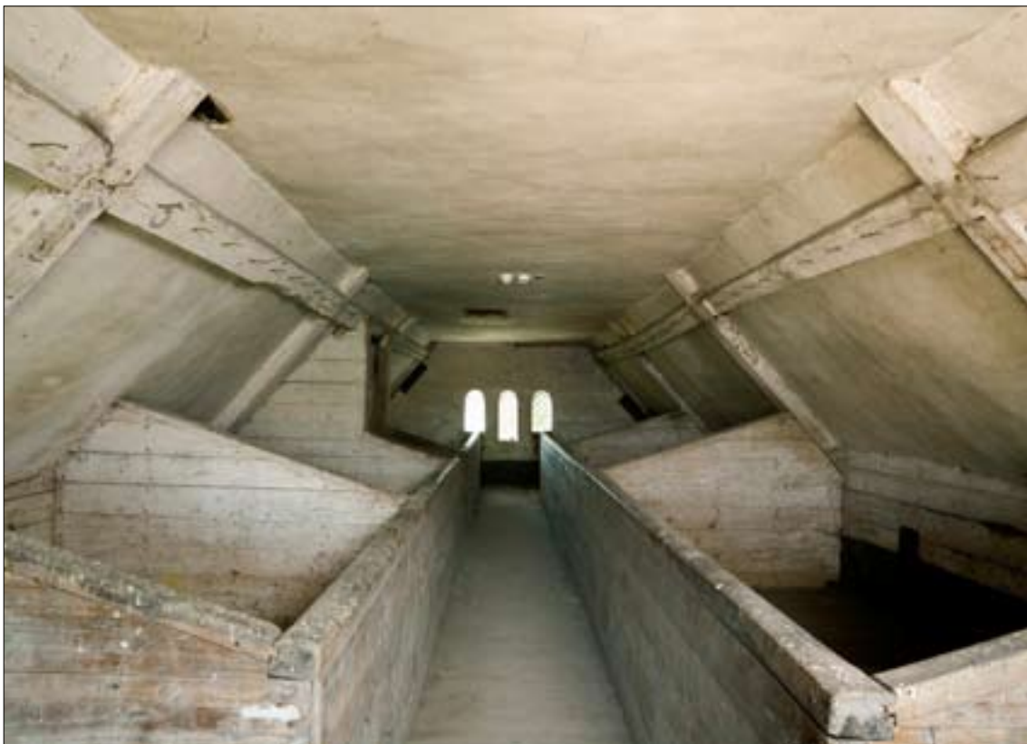
Fig. 33. The corn bins in the attic of the west crosswing, installed c.1777. © English Heritage DP029979
