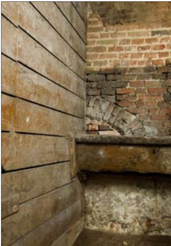
Fig. 16. The surviving blocked fireplace on the ground floor in the west crosswing.
