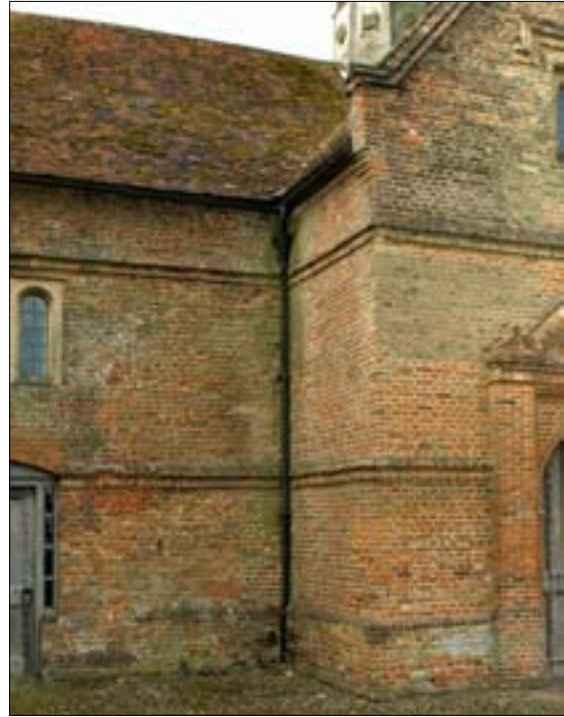
Fig. 26. The east corner of the central crosswing, where the lean-to addition once stood. © English Heritage DP029974
