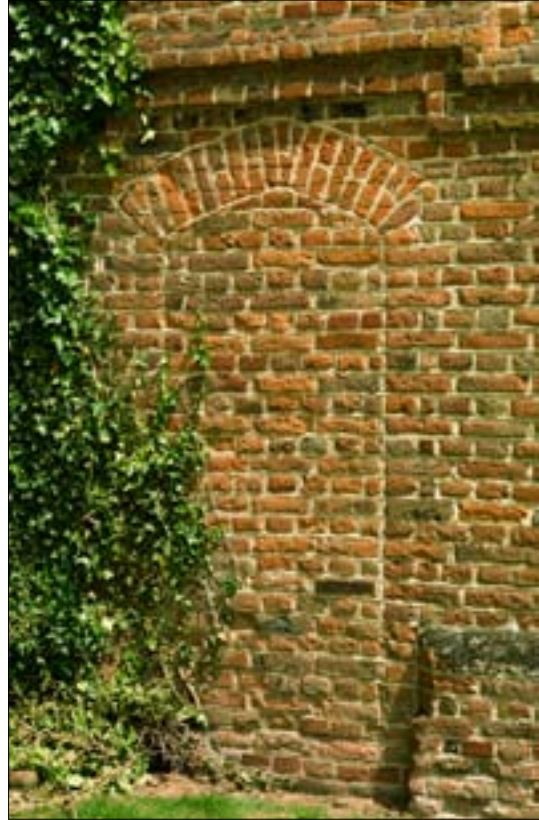
Fig. 6. The blocked doorway on the west return wall of the central crosswing, the south front.
