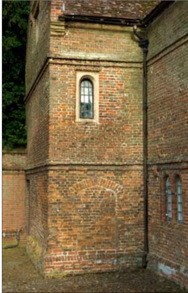
Fig. 9. The blocked doorway on the west return wall of the east crosswing and the former two light window above, now reduced to a single light window. © English Heritage DP029964
