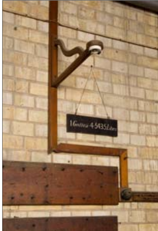
Figure 17 Timber electrical conduit, boards formerly carrying hooks for tools and signage. © English Heritage NMR DP070057
