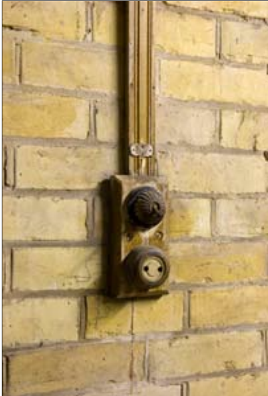
Figure 16 Light switch and socket for portable examination lamps. © English Heritage NMR DP070067
