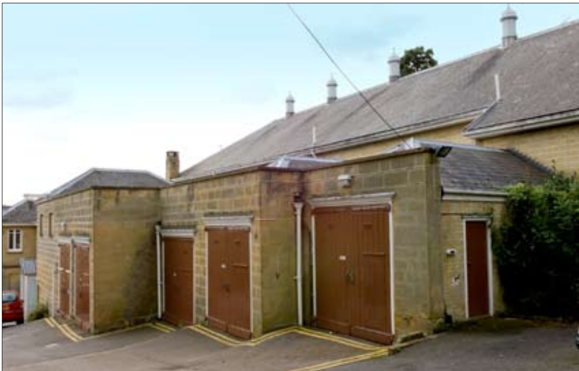
Figure 10 The motor stables from the north, showing brick construction exposed on the north wall.
