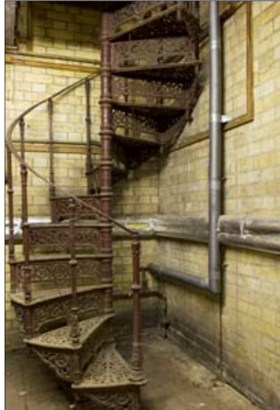
Figure 7 The spiral staircase rising from the basement level to garage 2. © English Heritage NMR DP070059
