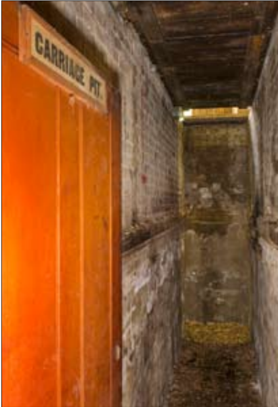
Figure 6 A motor pit showing the full height entrance doorway. © English Heritage NMR DP07066
