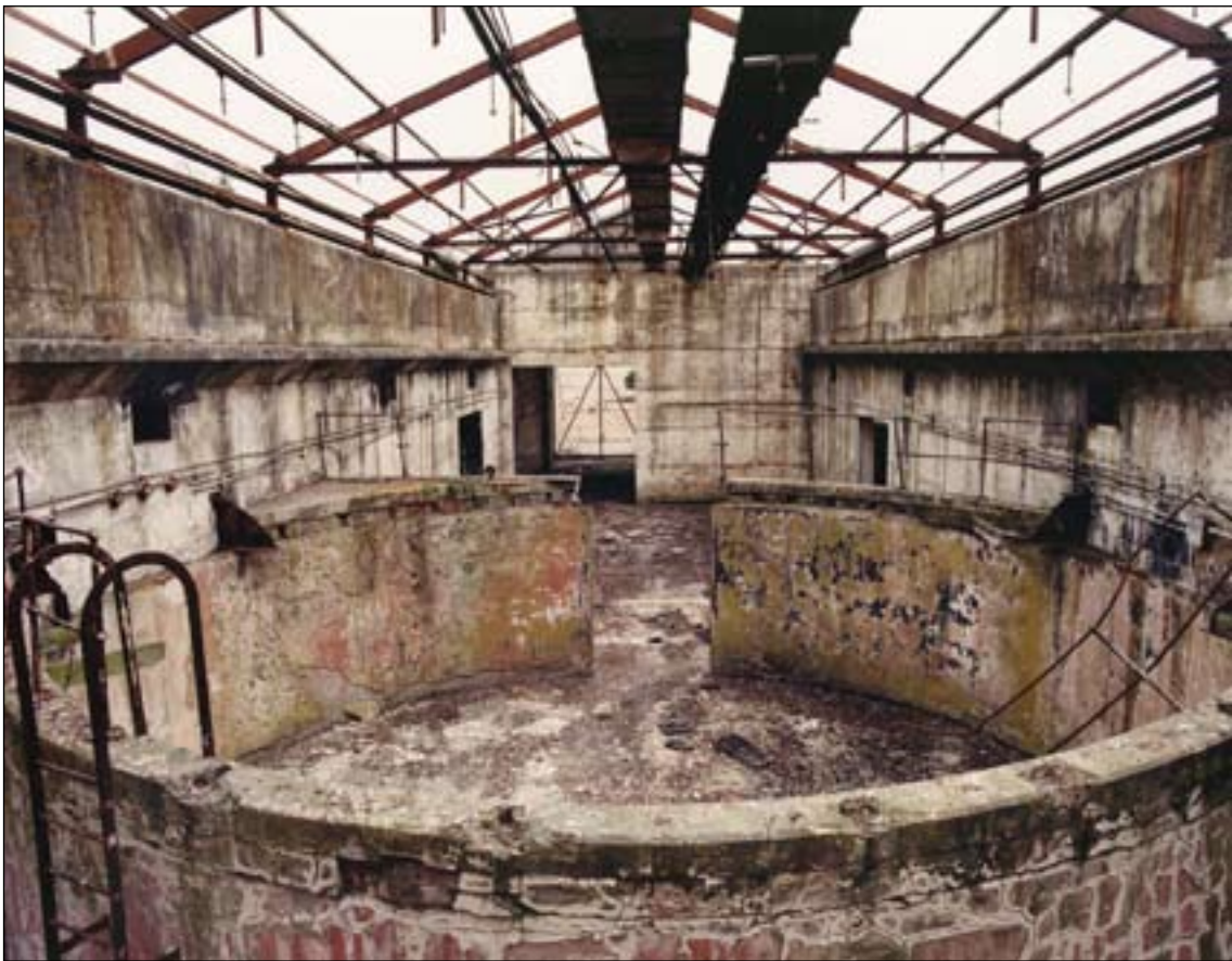
Figure 30: Laboratory I in June 2000, interior showing the centrifuge pit and above it a section of air conditioning conduit. Below the tops of the walls are projecting ledges that carried rails for a travelling crane. (c) English Heritage
