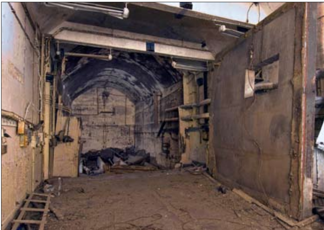
Figure 28: Laboratory 3, interior showing the rear climatic chamber and dismantled sliding door that sealed the chamber. (c) English Heritage DP068471
