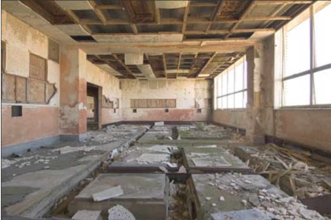
Figure 32: The Control Room E4, showing the large southwestern control room, with subfloor cable ducts and sound proofing boards. (c) English Heritage DP070006
