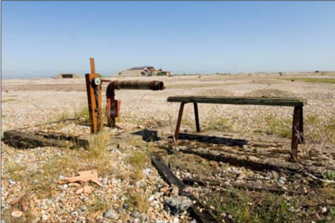
Figure 41: Fire hydrant. (c) English Heritage DP070008
