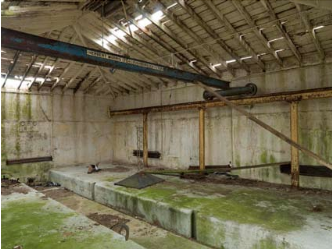
Figure 21: First World War Magazine D2 showing storage platforms and later alterations. (c) English Heritage DP070014
