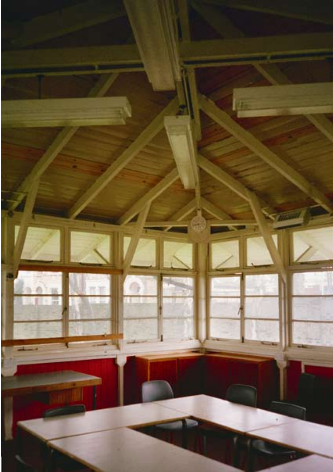
Frontispiece: Interior of pavilion classroom on the grade II listed Aspen House Open Air School, LB Lambeth (LCCAD, 1925) (DP070341).
