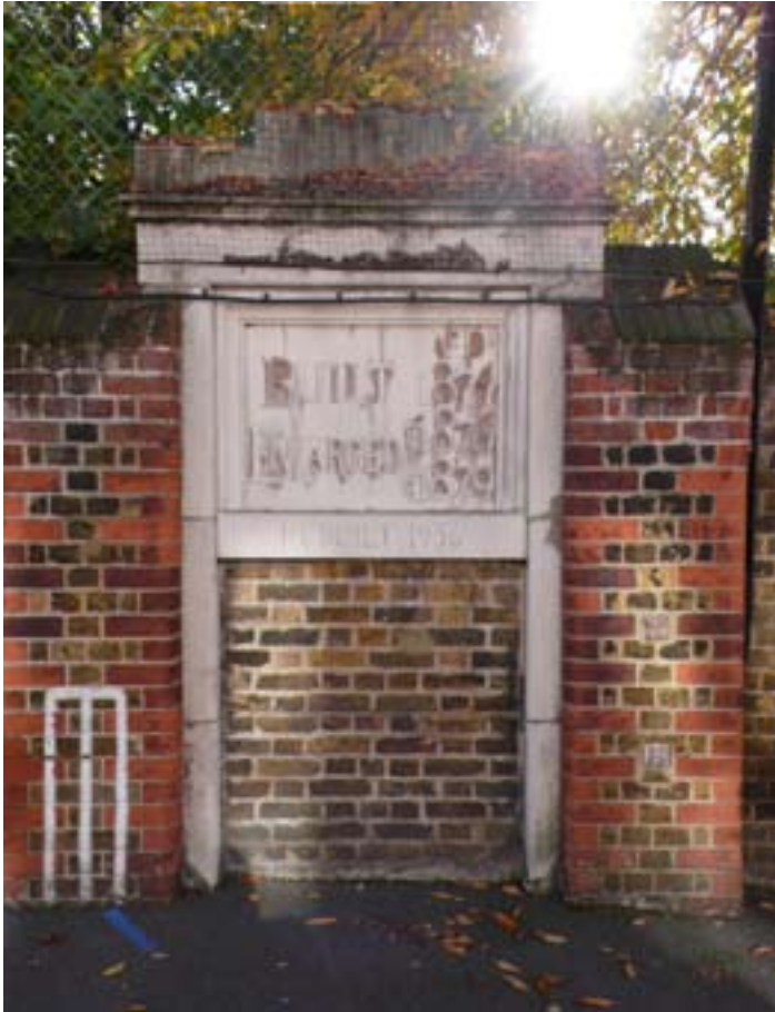
Fig. 12: SBL datestone from the West Kensington Central School, LB Kensington & Chelsea, reset in the boundary wall of the rebuilt 1936 school (DP070344).
