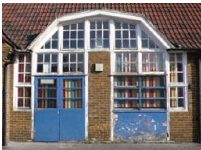
Fig. 4: Classroom lighting. Elaborate clerestory windows were employed by the LCCAD at Haimo Road, LB Greenwich (1925-26) and elsewhere (DP070343).
