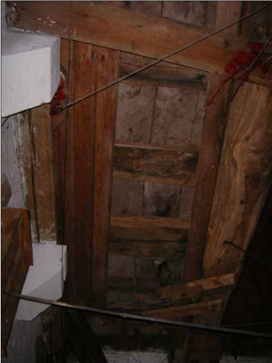
Figure 3: The underside of the belfry floor, primary beam 4 is against the wall to the far left of the photograph
