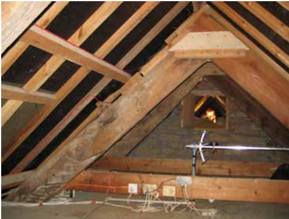
Figure 6: The east principals of Trusses 2 and 3 of the roof over the West Wing viewed looking south-east
