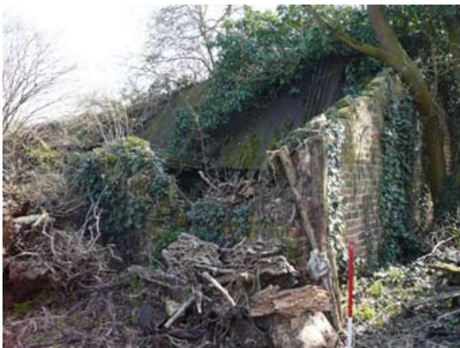
Plate 11: Partly collapsed tool shed/fruit store at the north-western corner of the walled garden © David McOmish
