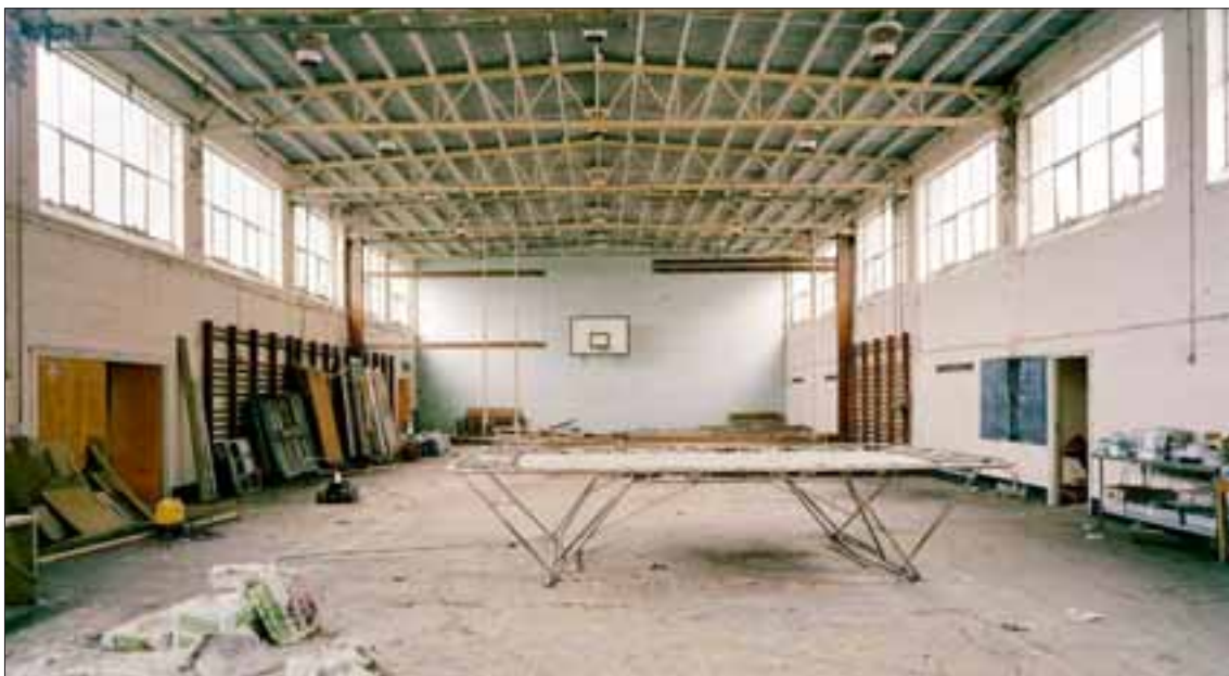
Fig. 23 The abandoned gymnasium.
