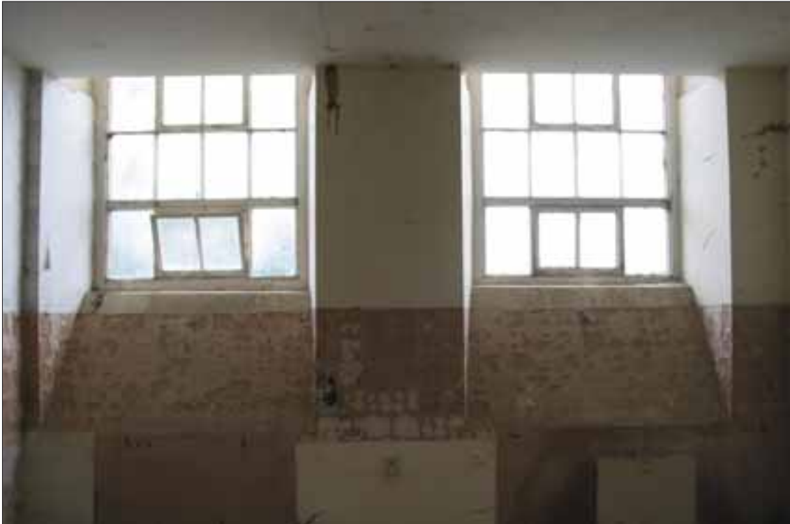
Fig. 14 Metal framed windows in the Orangery, showing the depth to which the floor has been lowered.
