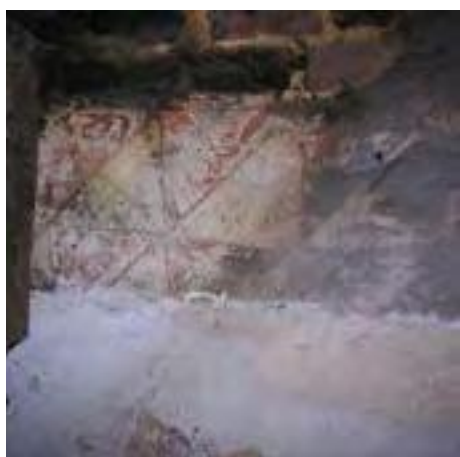
Fig. 17: Traces of a geometric decorative scheme of probable 17 th century date surviving on the plasterwork lining of the hall fireplace jamb. (DP040085).
