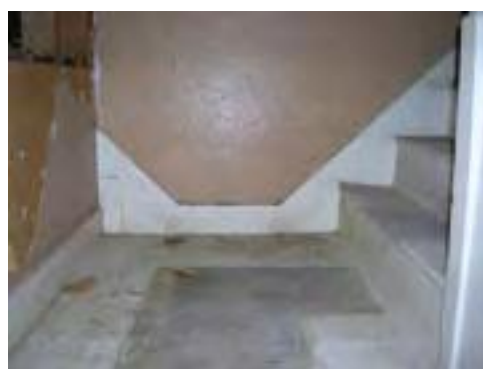
Fig. 52: The back stair originally divided into two short flights of three steps, leading into lobbies to the north and south (DP070338).
