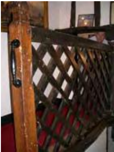
Fig. 58: Lattice balustrade to stair in East End Farm, Cottage, Pinner (© Patricia A. Clarke).
