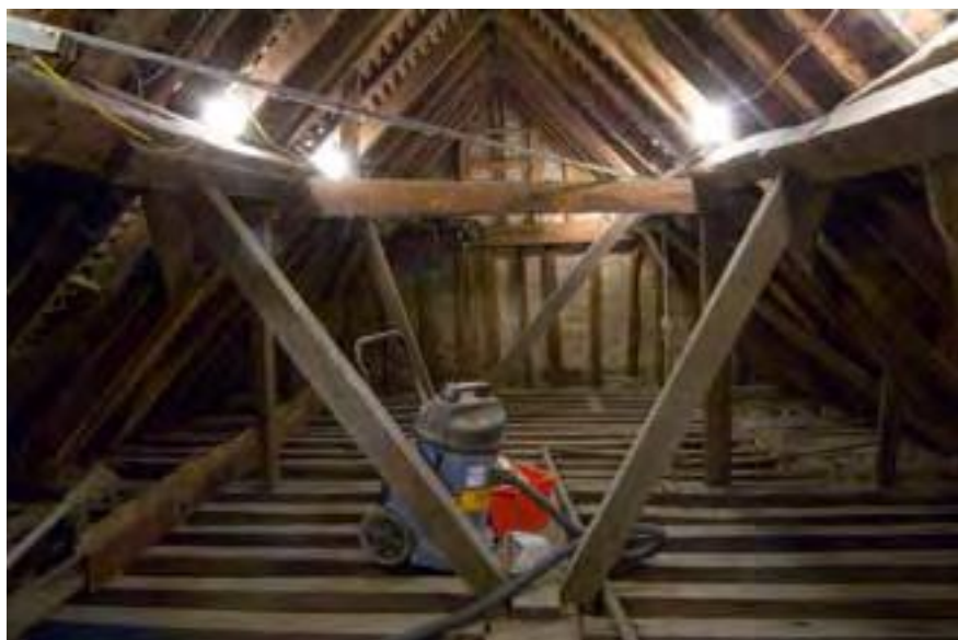
Fig. 35: Roof space of hall range, looking north. The struts in the foreground are later insertions. Photograph by Derek Kendall (DP042418).
