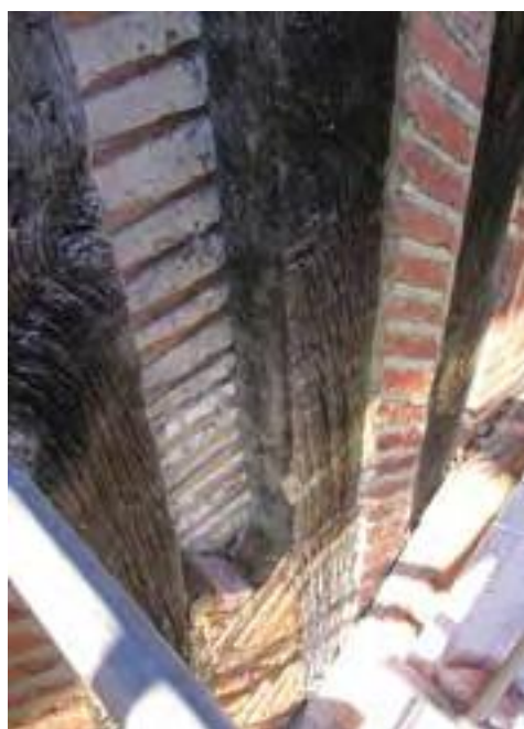
Fig. 9 The partial removal of nogging during conservation works in 2007 showed that the reveals of the studs were hollowed to provide a mortar key (DP040076).
