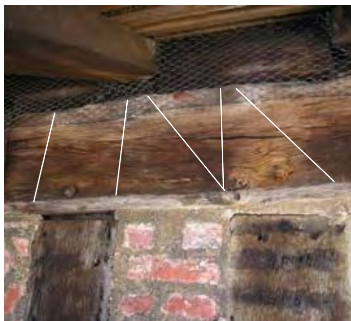
Fig. 10: Scribing marks on the wallplate of the west elevation (highlighted in white), inscribed during the 'setting-out' of the timber frame to indicate the position of the adjoining studs (DP040078).
