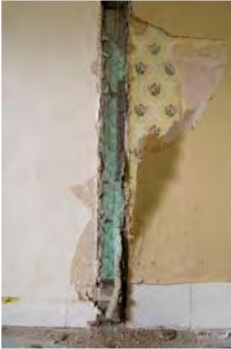
Fig. 64: Wallpaper fragments discovered in 2007 on the north wall of the hall chamber when partitions formerly dividing rooms 23, 31 and 32 were removed. Photograph by Derek Kendall (DP042394).
