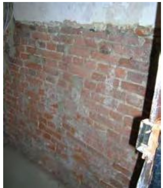
Fig. 57: East wall of room 12 (west wall of principal stack) exposed during works in 2007-08. Note inserted, and subsequently blocked, sockets for stair risers. (DP0070339).
