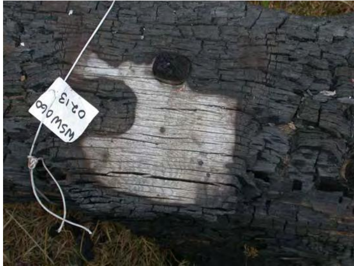
Figure 11. Charred and unburnt wood from the underside of a beam.
