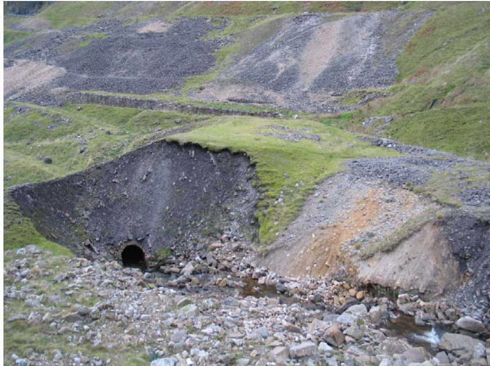
Figure 4 Erosion of waste heap 41 over culvert 35 and the surrounding area (taken in November 2006)
