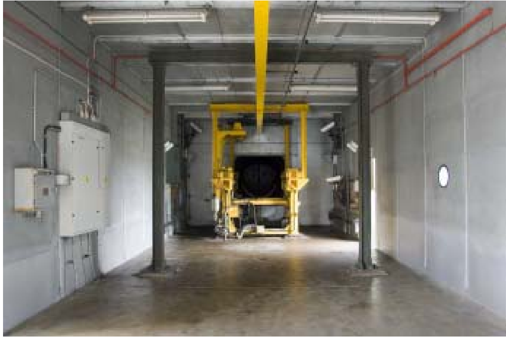
Figure 163 Uninstalled Engine Test Facility (UETF), test chamber looking towards the mouth of the detuner, which reduced the noise during test firing. (c) English Heritage DP027325
