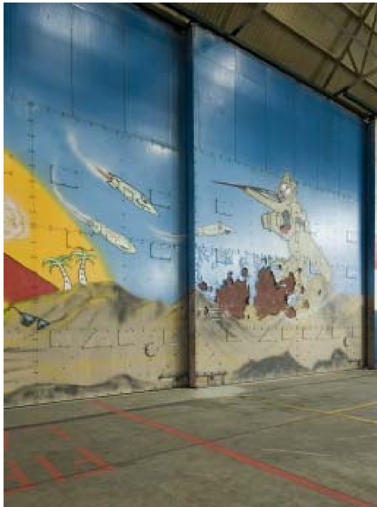
Figure 209 October 2006, Hangar 1 east doors detail of painting showing deterioration of the paint work a few months after the RAF's withdrawal. (c) English Heritage DP035655
