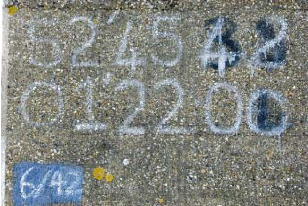
Figure 259 Late 1950s blast protection wall, the numbers refer to the bearing of the shelter's centre line, allowing the aircraft's navigation aids to be set prior to take-off. (c) English Heritage DP027326
