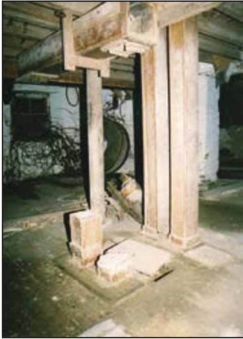
Figure 20. Interior, first floor of mill, from south east, showing elevator casing, aspirator trunking above, and a millstone in the background. To right is the doorway into the north extension. [OP04337]
