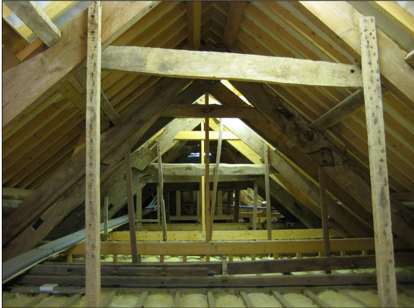
Figure 5: North-south range, showing the empty mortices for collars and through purlins in the principal rafters, looking north
