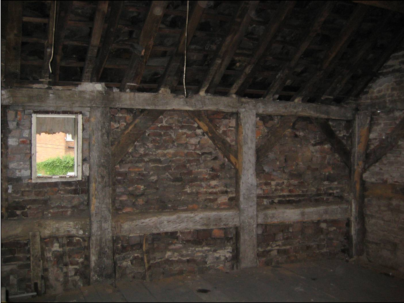
Figure 6: Northern range; first-floor framing in room F25, photograph taken from the south-west
