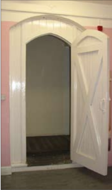
Figure 9. External door reset in an internal doorway.
