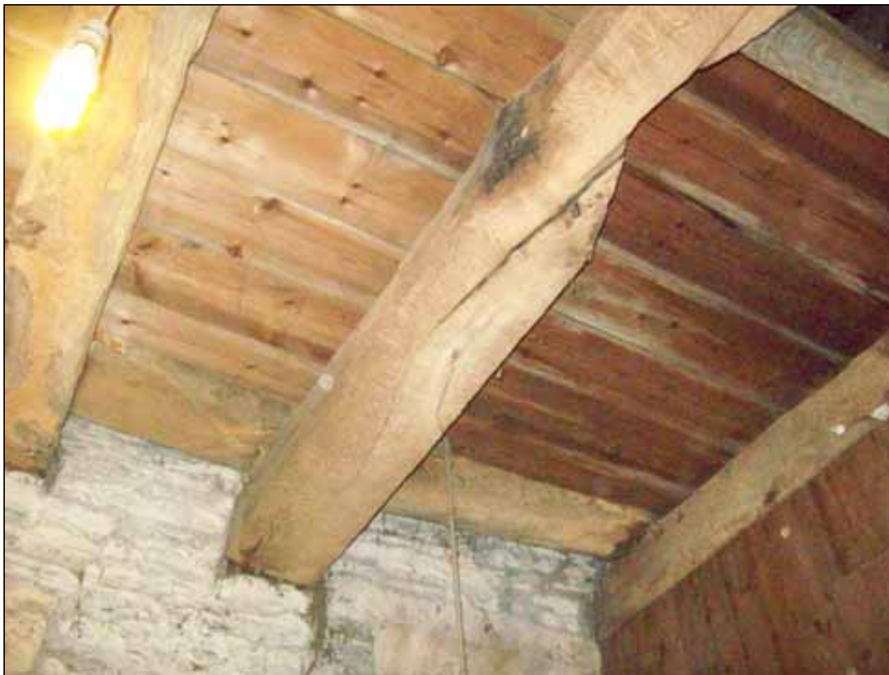
Figure 6: Belfry floor, beam 4 to far left and west bearer in towards the rear
