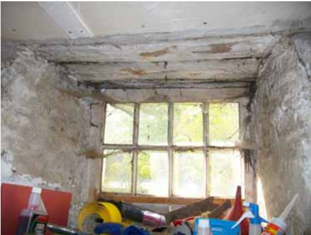
Figure 5a/b: Cruck truss (top) and window lintels (bottom) to the 'museum wing'
