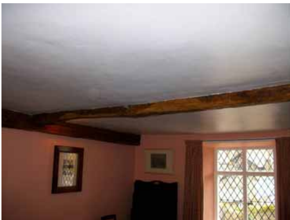
Figure 4a/b: Ground (top) and first-floor (bottom) ceiling beams of the house range
