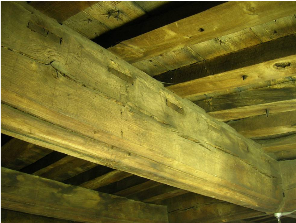
Figure 4: Empty mortices and reset common rafters to the south pitch of the lower roof
