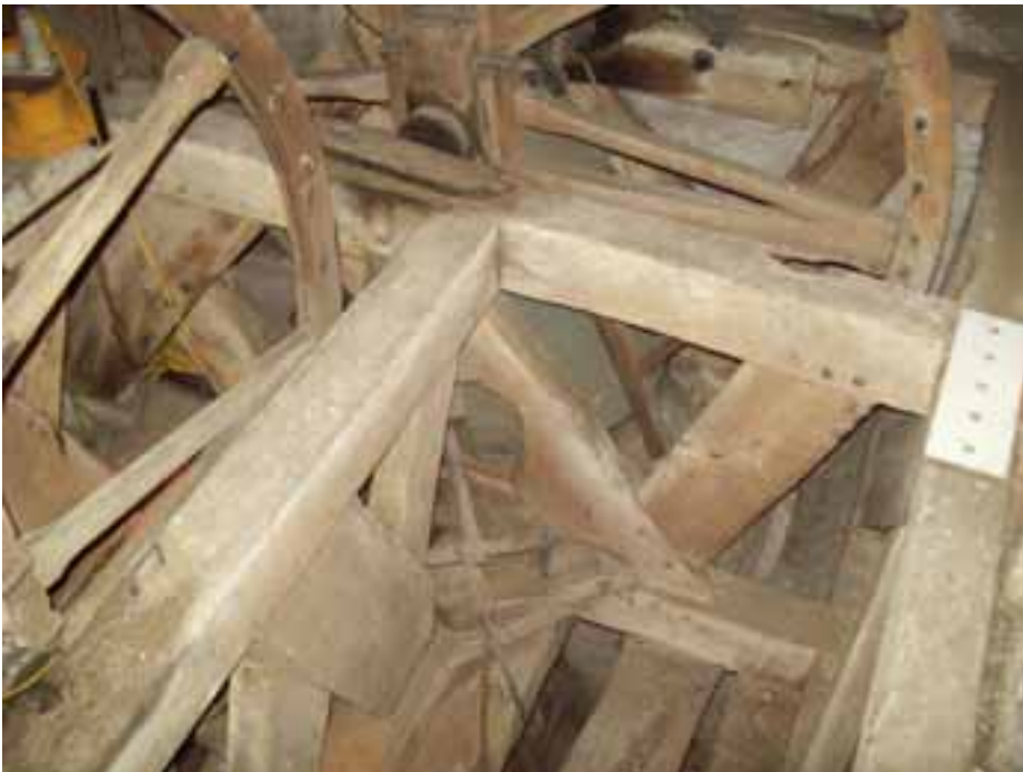
Figure 6 (top): View of the beams to the floor of the winding chamber
