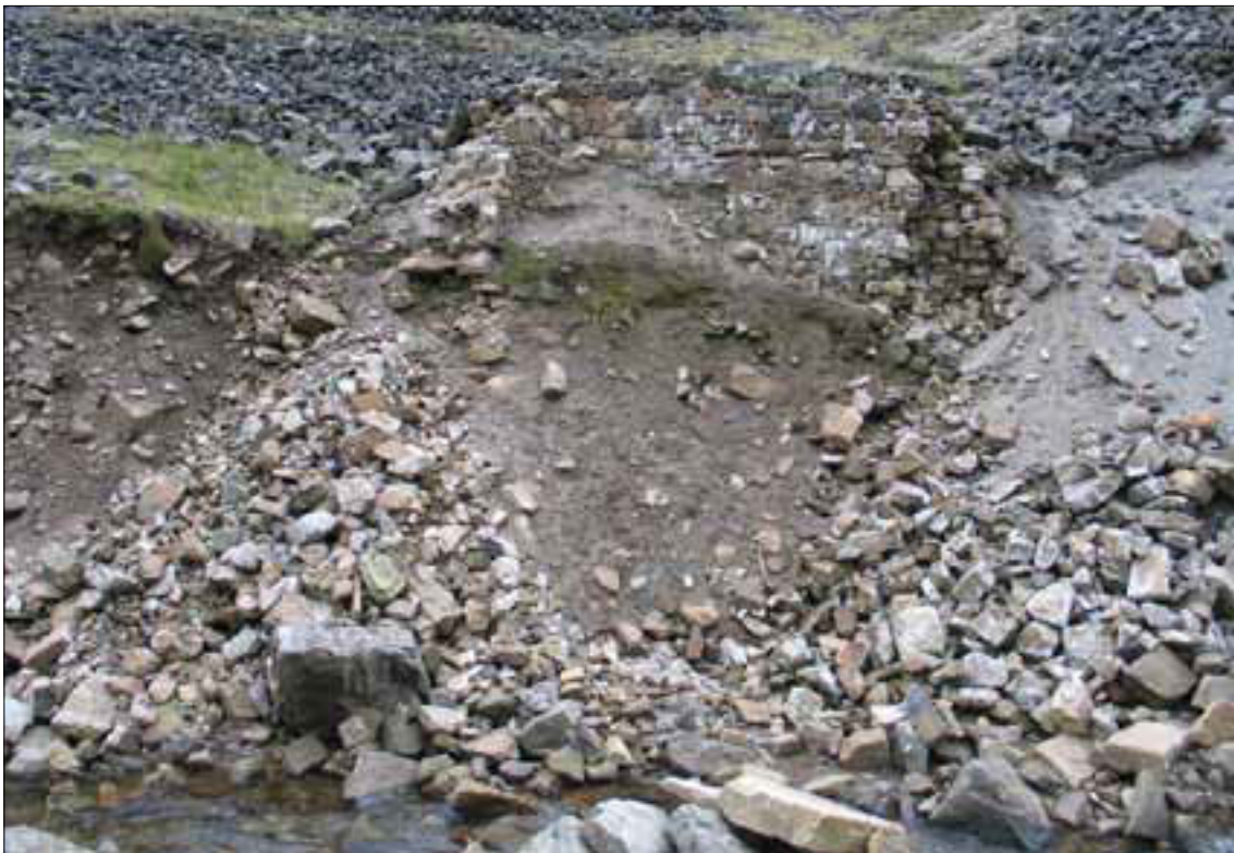
Figure 56 Remains of possible ore store (78), adjacent to Scordale Beck. All that survives of the structure is the rear wall and part of one of the side walls - the rest has been lost to erosion.
