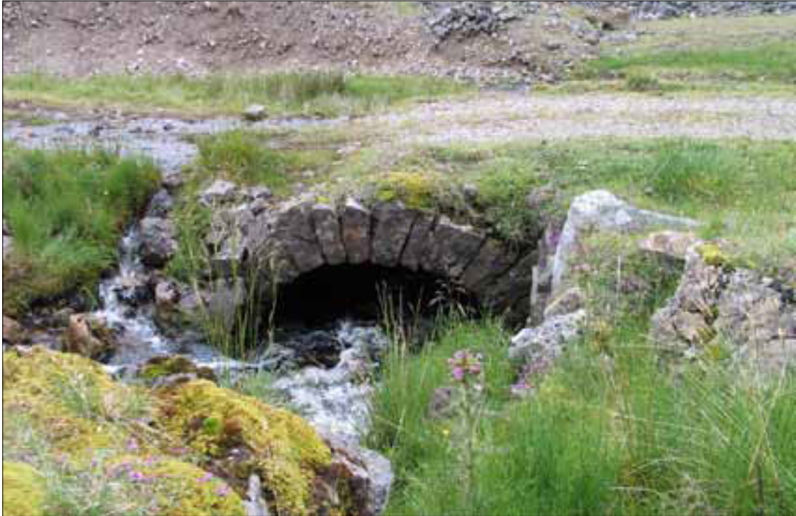
Figure 64 Culvert (33) carrying the mine road (32) across Stow Gill. Water flow off the road and from Stow Gill is causing erosion to this feature, visible to the left of the arch in this photograph
