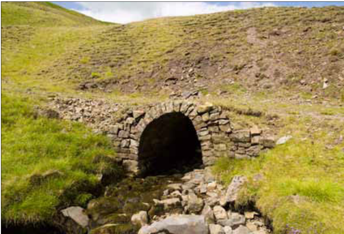
Figure 63 The culvert (35) carrying the main mine road (32) over Scordale Beck. The large mass of material on top of the culvert is a spoil heap (41).
