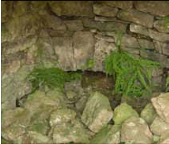
Figure 95 The surviving draw-hole in the rear wall of the chamber of limekiln 623
