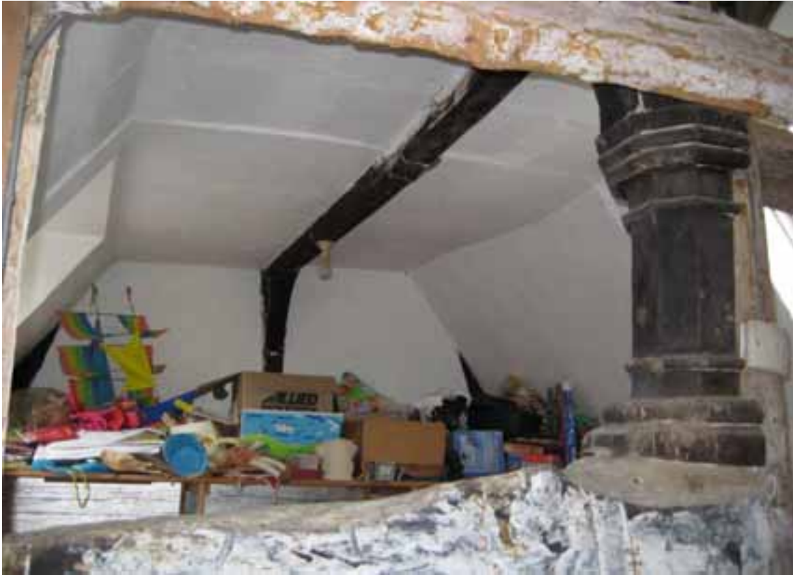
Figure 5: Crown post of Truss B with Truss A in the background, viewed looking south-east
