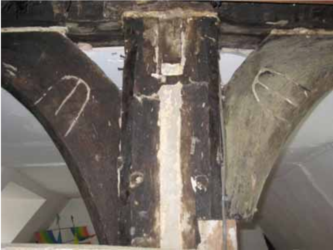
Figure 7: Detail of the Arabic assembly marks on the west face of the upward braces from the Truss B crown post to the upper crucks viewed looking east
